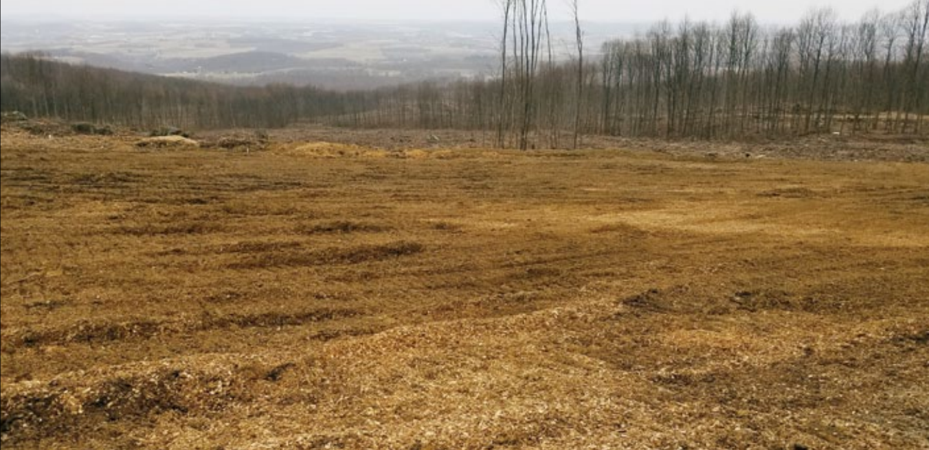
A large landing area (foreground), covered in wood chips, helped to prevent erosion and sediment pollution during a landowner's forest clear cut (background) in Mount Pleasant Township.
