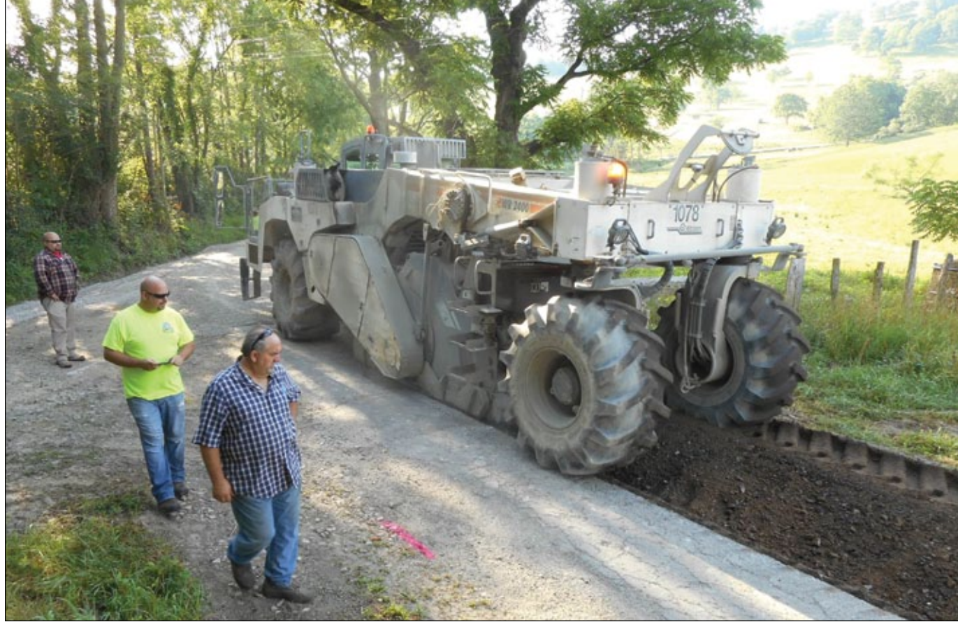
A "reclaimer" mills the existing asphalt and base materials on Hartman Road during the first full-depth road reclamation in Westmoreland County.
