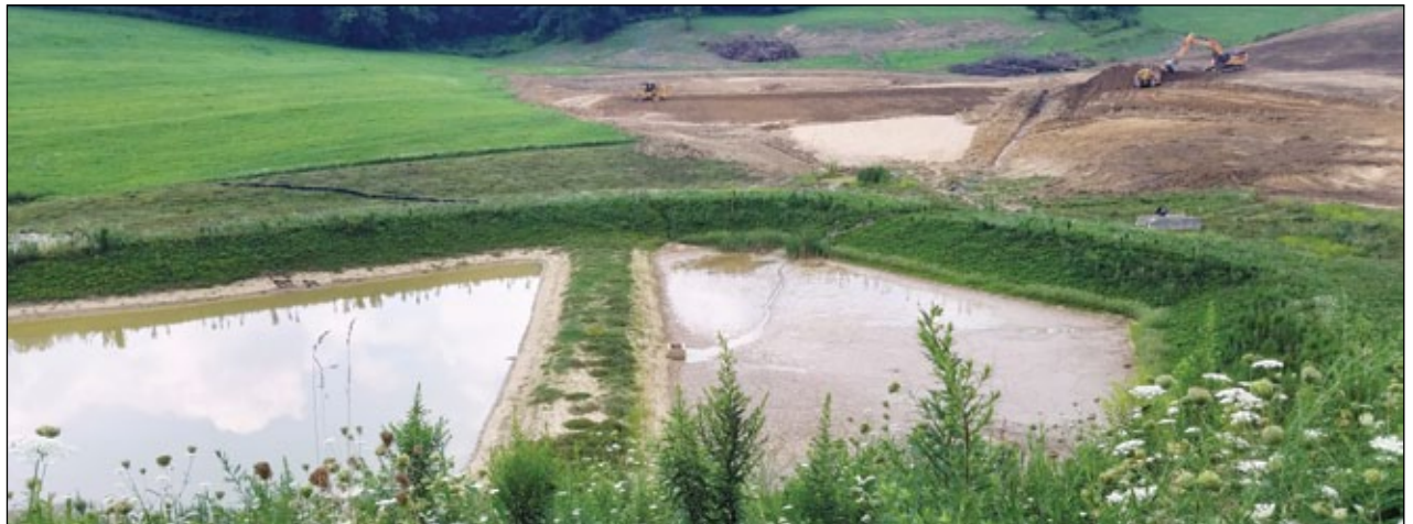
Continuing development of North Huntingdon's Tuscan Hills residential plan included creation of a forebay (right, foreground) and sediment basin (left, foreground) for temporary erosion control and permanent stormwater control.
