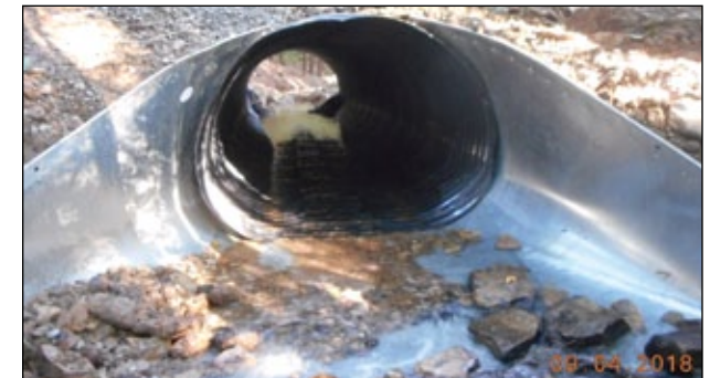
“Squash pipes” were the perfect replacement for two badly deteriorated 36-inch pipes that carried an unnamed tributary under Sugar Run Road in Saint Clair Township because they could contain the entire seven-foot width of the stream without having to markedly raise the road profile.
