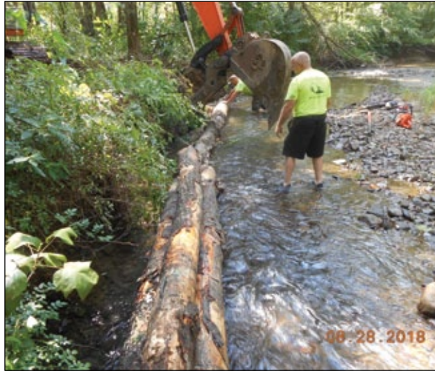
Improvement work on Jacobs Creek, just upstream from Bridgeport Dam, involved installing stacks of logs along some 1,200 feet of the stream edge to reduce erosion and create habitat for fish.
