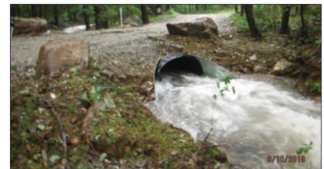
One of the new squash pipes doing its job after a heavy rain six days after installation.
