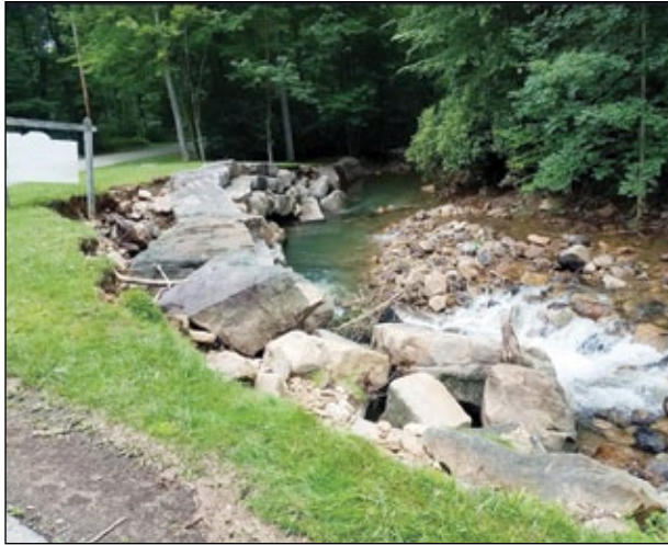
A look at Linn Run downstream from the Valley School of Ligonier shows the damage left behind by the high, swift floodwaters – the large amounts of sediment deposited on the right side of the stream; the severe undercutting of the streambank (behind boulders) on the left side of the stream.
