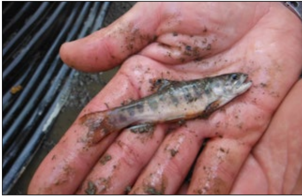
Native brook trout now have an easier time travelling in Poplar Run, thanks to a new, wide drainage pipe installed level with the streambed. The drainage pipe installation was part of work done to improve water quality along a section of Sugar Run Road.
