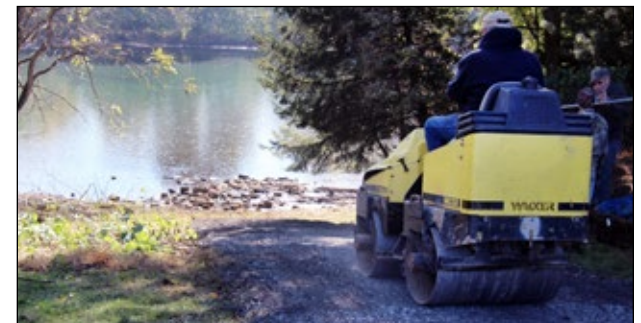
As water quality in the Kiskiminetas River improves, the number of recreational canoeists and boaters grows. To provide better access to the river and reduce erosion, we worked with the local watershed association to install a hard-surface ramp to the water.
