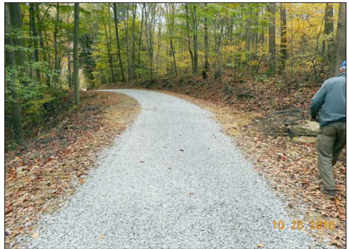
The road after construction was completed; note how the road is no longer entrenched
