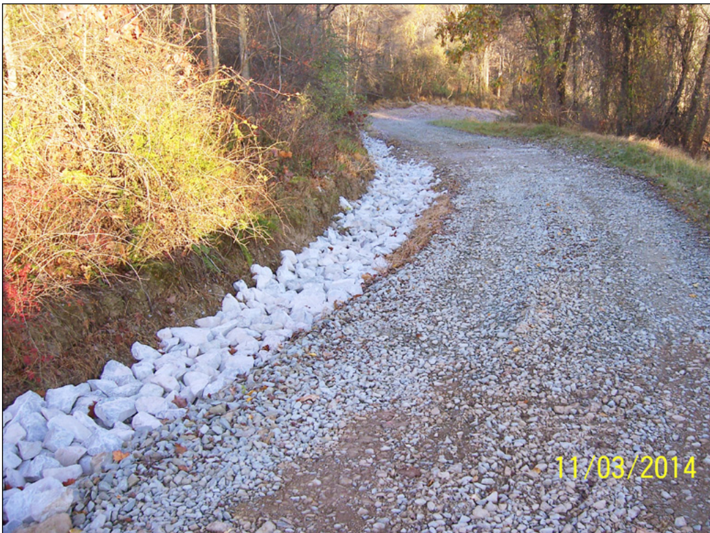
A similar section of road after underdrain was installed and the berms were removed
