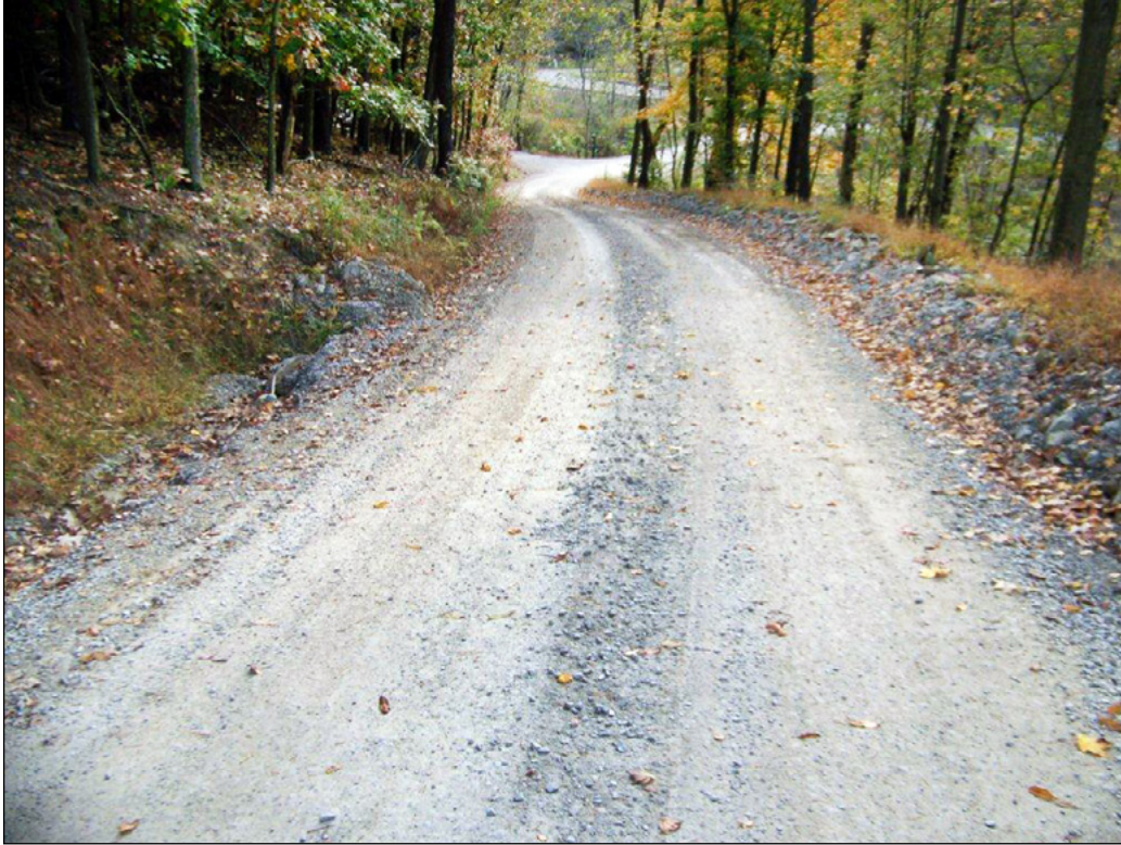
A section of road around Beaver Run Reservoir before construction; note the berms on the side of the road that held water in the roadway
