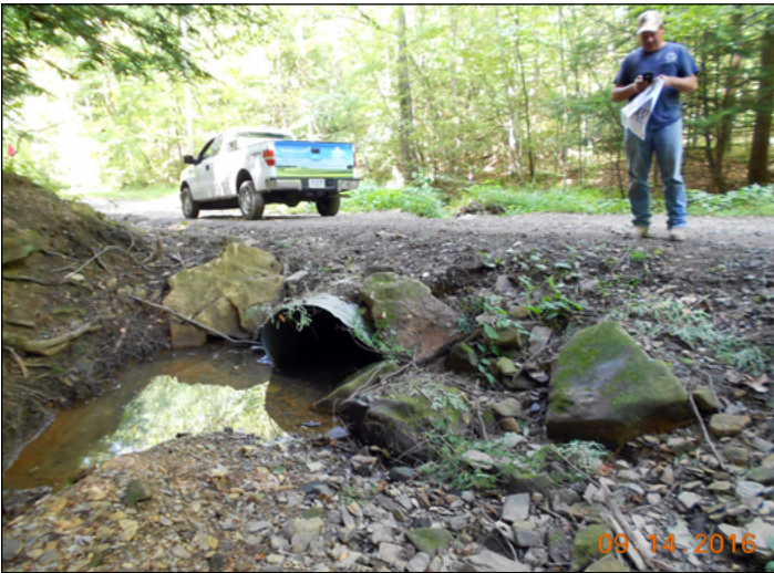
Coal Hollow Road before construction; note the lack of headwall and overflow pipe
