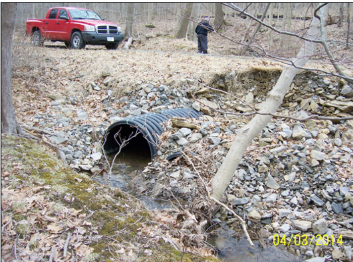
Another section of road around Beaver Run Reservoir; the crosspipe was installed incorrectly and needed to be realigned to remove the 90 degree bends at the inlet and outlet of the pipe
