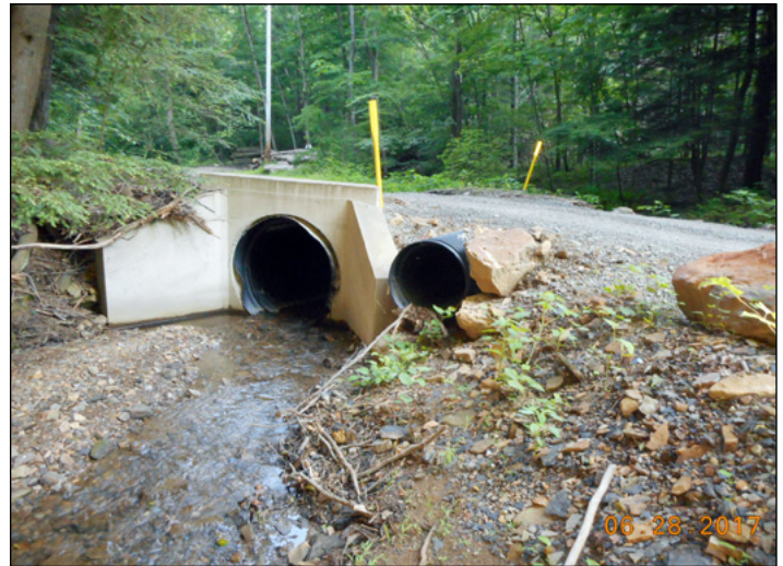
The same section a year after construction; a headwall and overflow pipe were installed along with a new crosspipe
