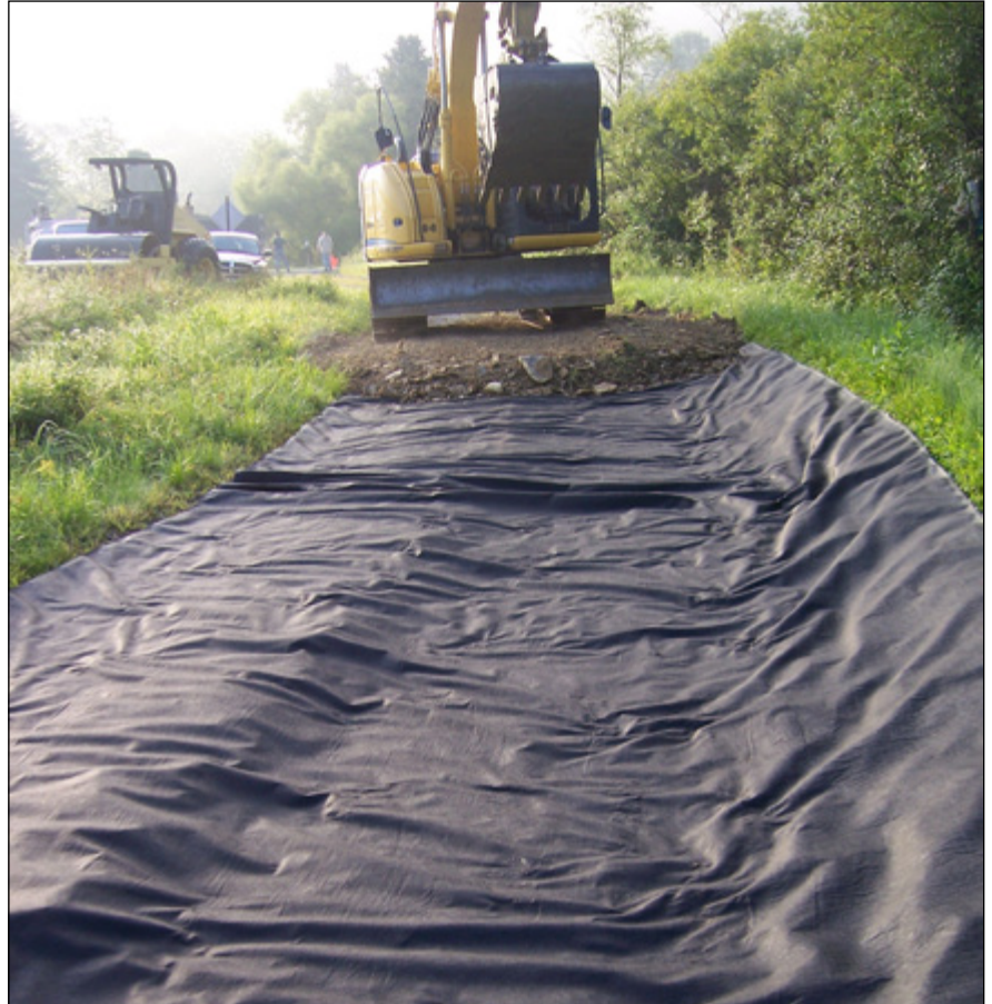
Placement of Geotextile fabric under road fill, to allow water to pass through and provide surface strength.
