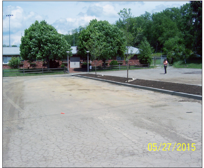
The new curbed rain garden with curb cuts, trees, and native seed mix
