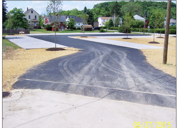
The tennis court area after the permeable parking lot with an asphalt driving lane and turfstone parking spaces was installed
