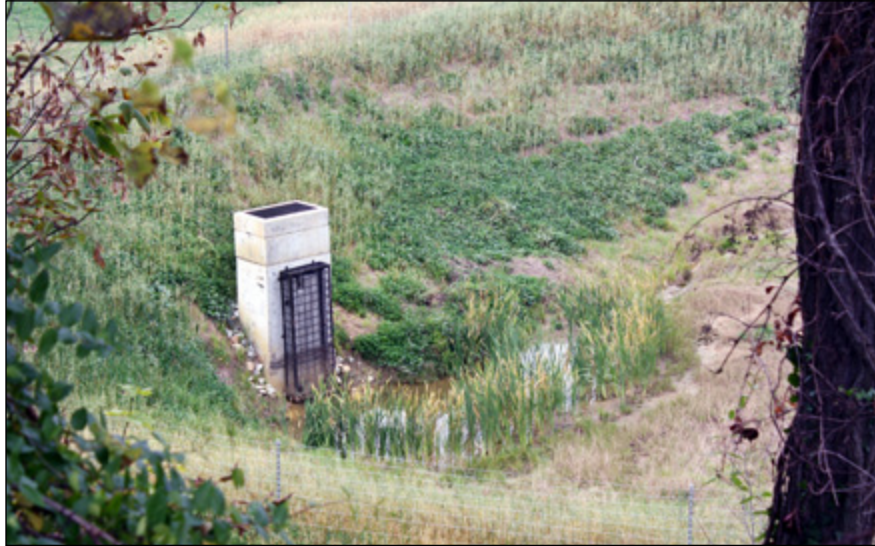
Water quality basin micropool at outlet riser allows pollutants to drop out before leaving the basin
