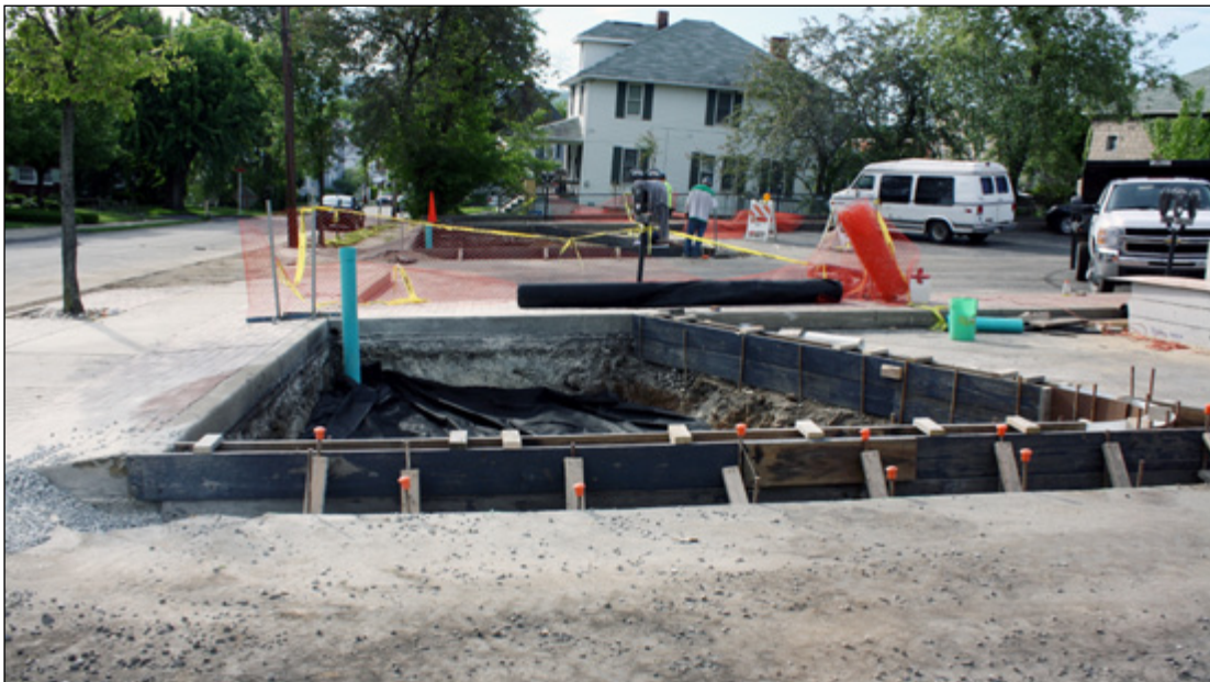
Concrete curbs with formed curb cuts protect the rain garden from traffic and allow water into the rain garden. A gravel underdrain is separated from the soil layer with a geotextile and a pipe riser will handle overflow in large storms.
