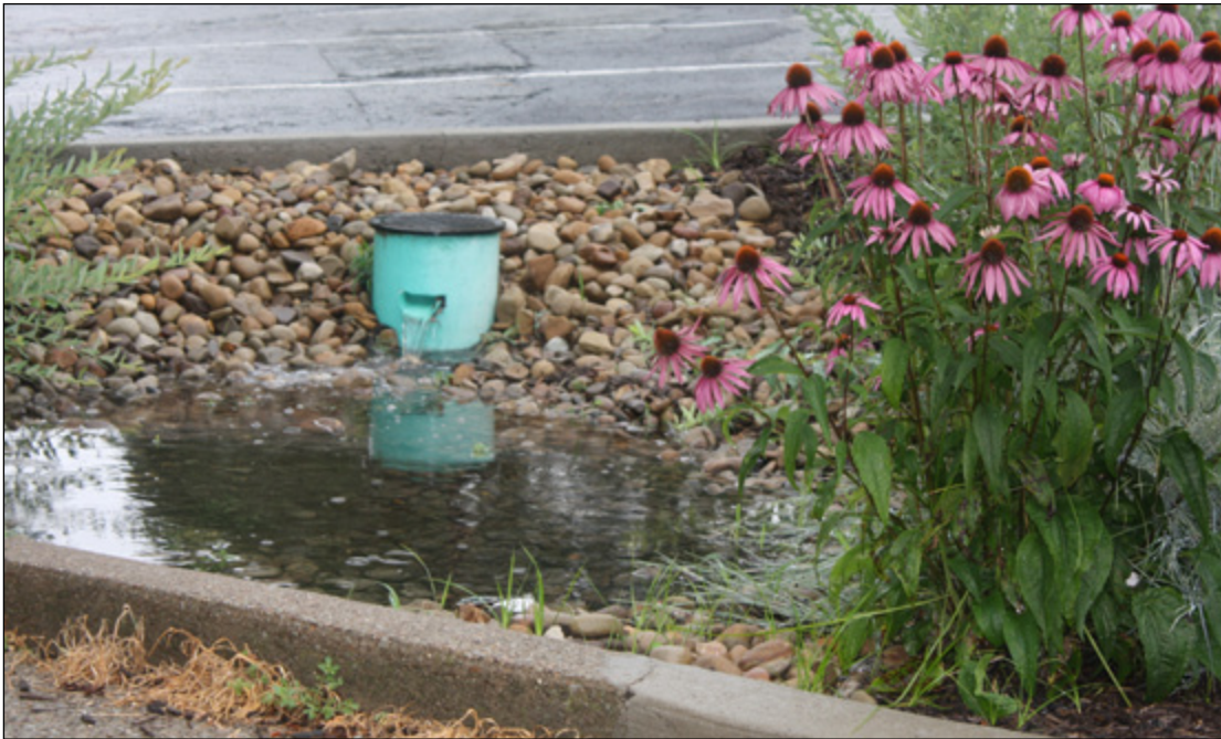
Runoff captured in the parking lot trench drain is reduced by a flow splitter to safeguard overloading a rain garden already limited in size by existing conditions.
