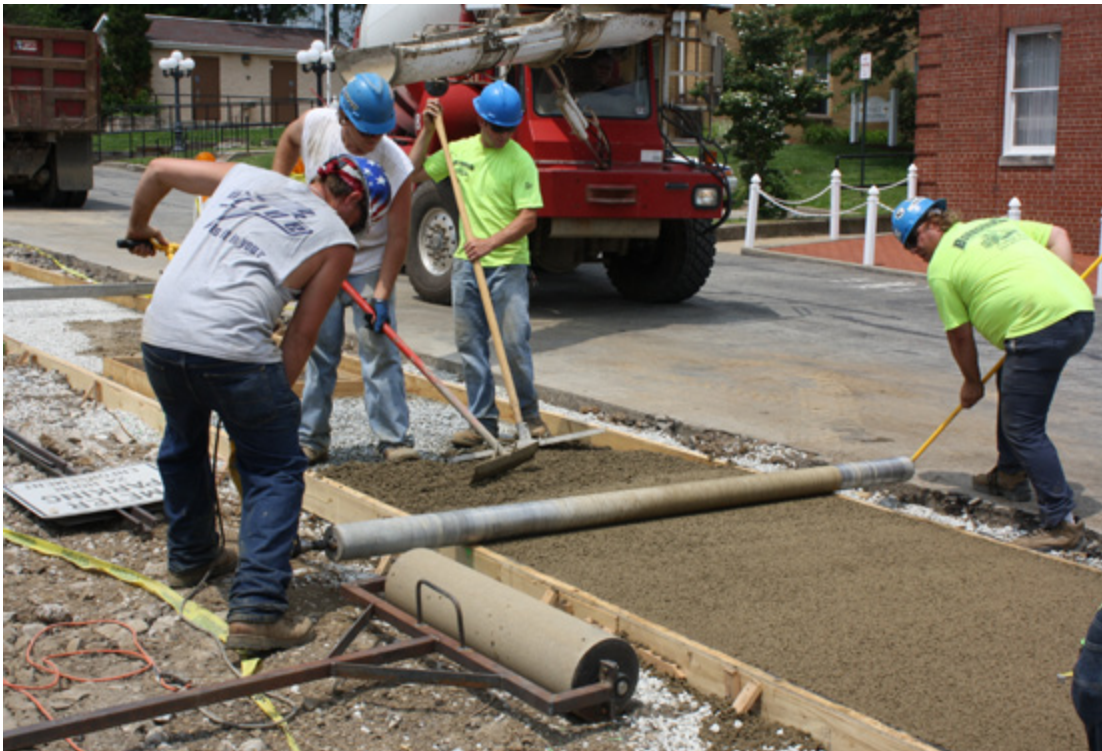
Permeable concrete is poured flush with the surrounding parking lot to handle stormwater.
