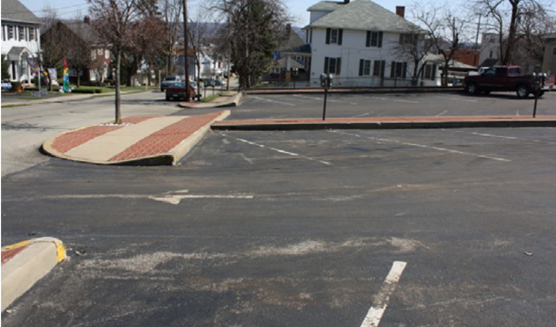
Mount Pleasant Borough Parking Authority lots generated uncontrolled runoff into the Borough streets and onto neighboring properties prior to the rain garden project
