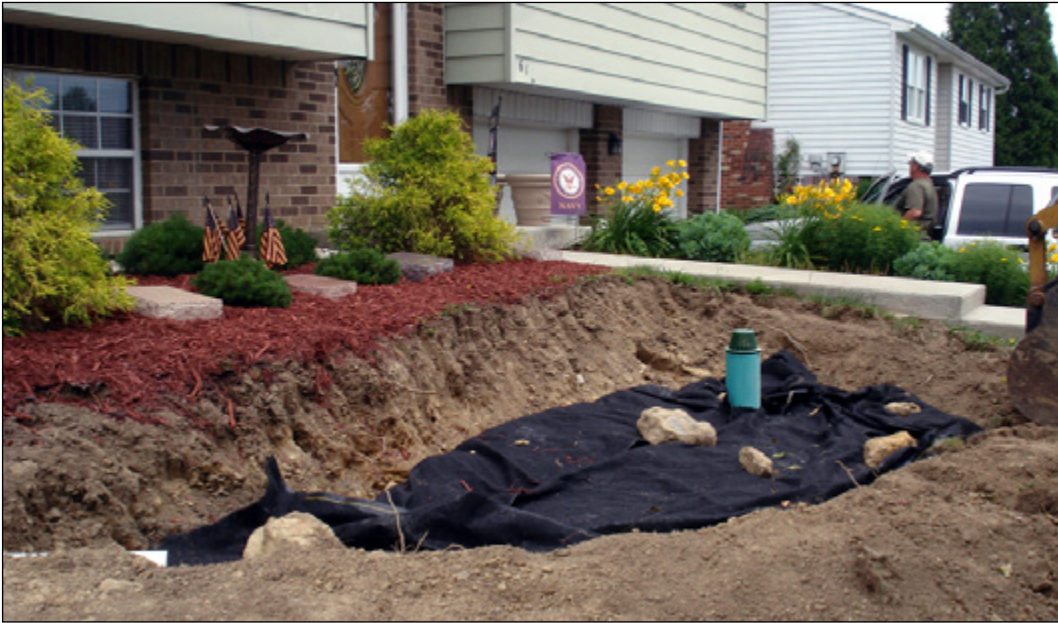
An underdrain layer is separated from the soil mix with a geotextile, and a pipe riser extends up to capture excess runoff from large storms.
