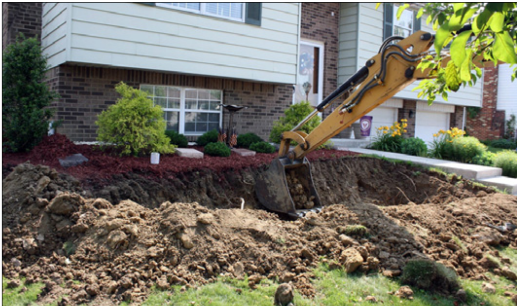
After verifying no utilities are in the way, a rain garden is excavated three to four feet deep to allow for an underdrain and soil mix layers as well as surface ponding depth.
