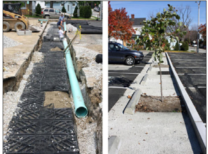
Trenches were cut and excavated across a parking lot and filled with a soil containment system, covered with permeable concrete and planted with trees.
