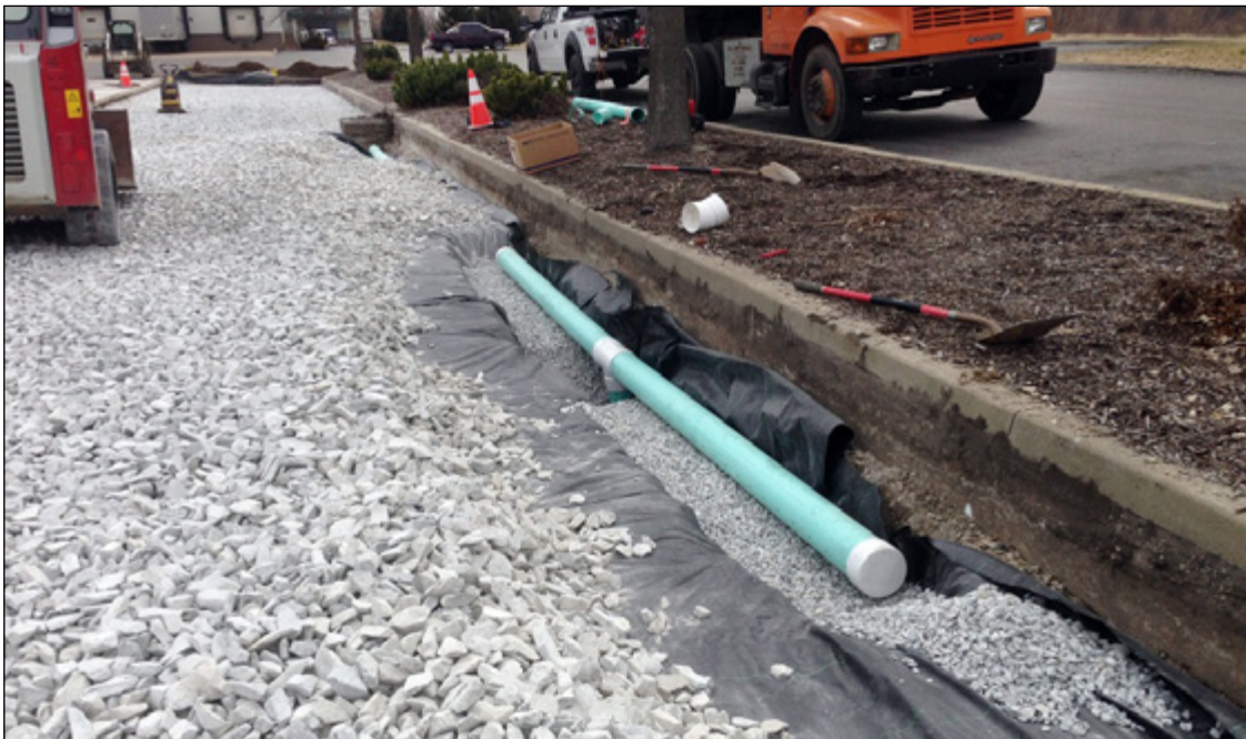
A perforated underdrain beneath the pavement takes excess runoff from large storms away from the infiltration system.
