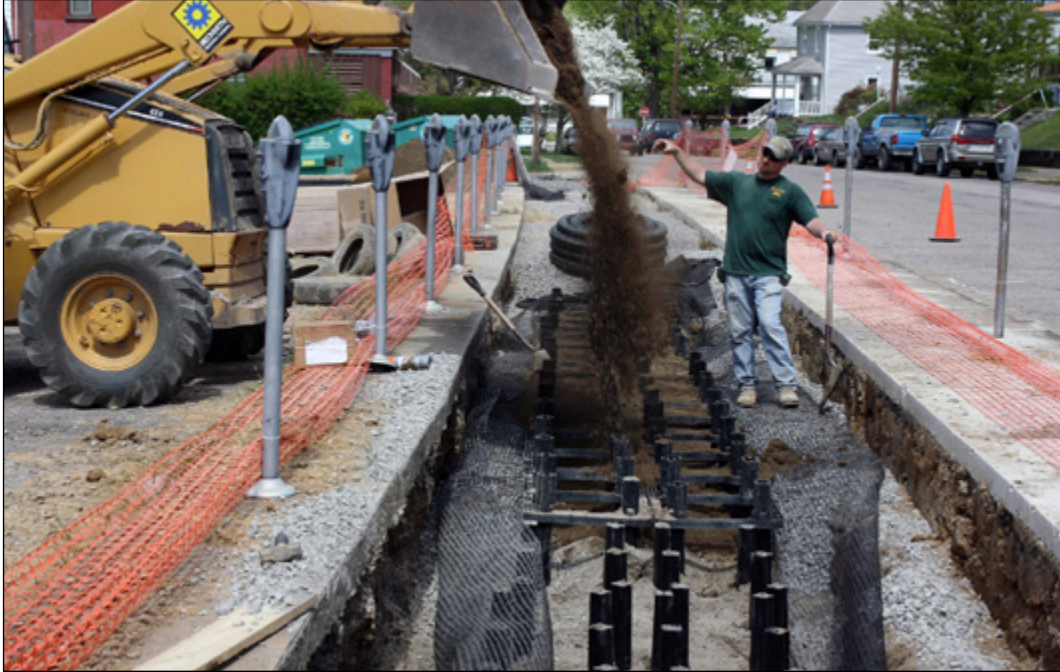
Soil containment system being filled with an engineered soil mix to support tree root growth beneath new permeable sidewalk.
