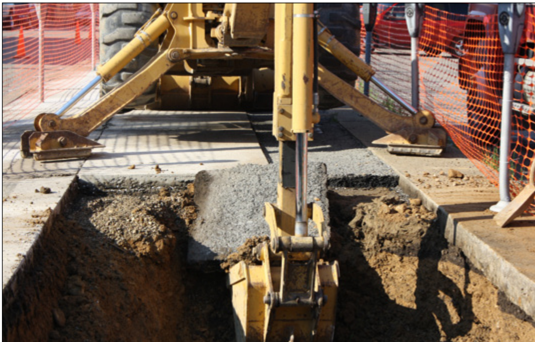
Existing sidewalk pavement was removed and 4 foot deep trench excavated to provide the depth for the soil containment system to capture and treat stormwater runoff.
