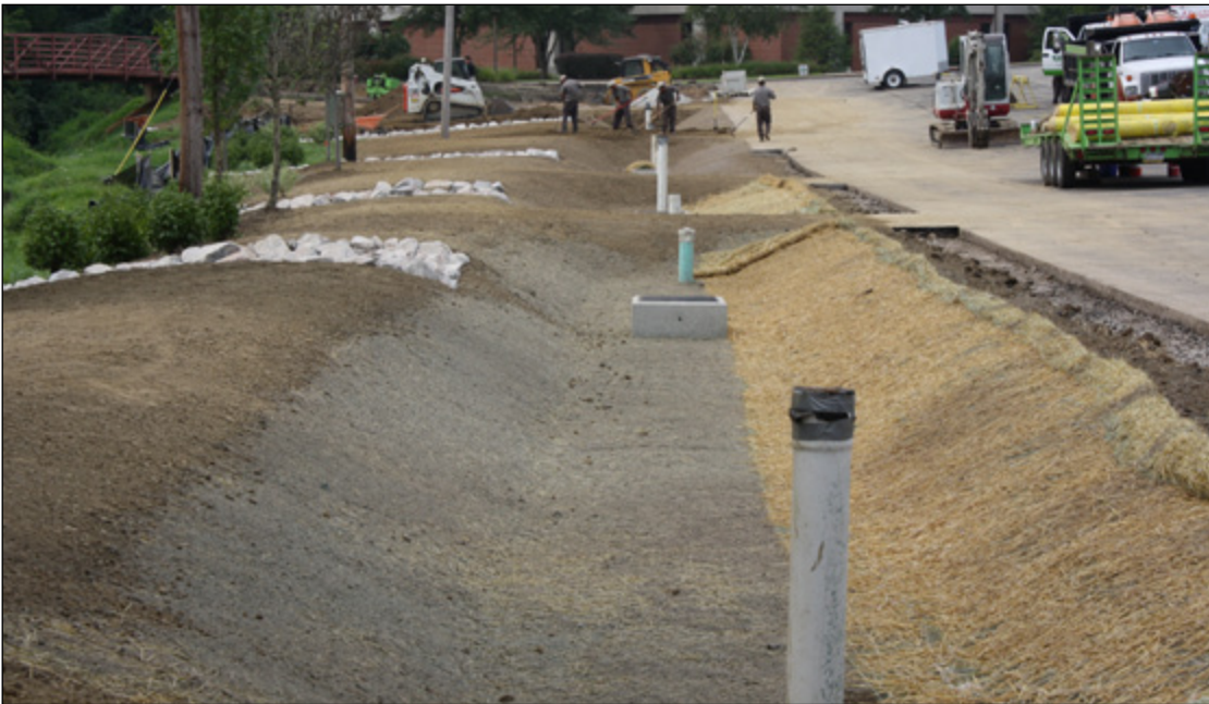
Four infiltration trenches were installed over underdrains to capture debris and allow surface runoff to infiltrate. The leading edge was protected with a concrete strip and a turf reinforcement mat.
