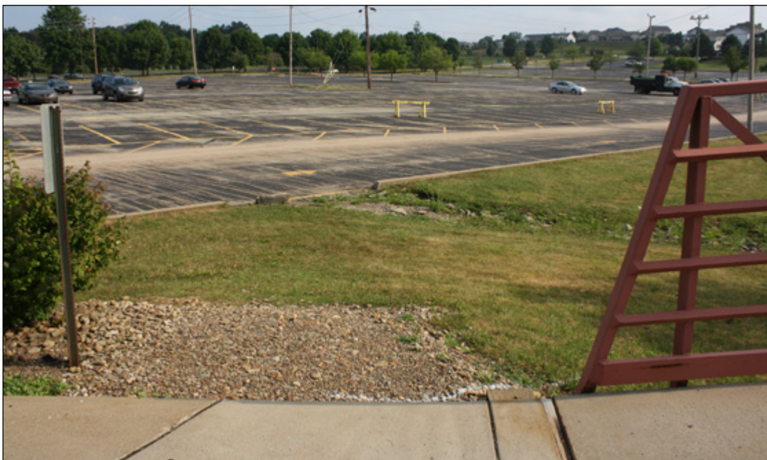
Looking up across the existing 4 acre parking lot from a pedestrian bridge, showing the eroded channel from surface runoff concentrating on its way to the stream.
