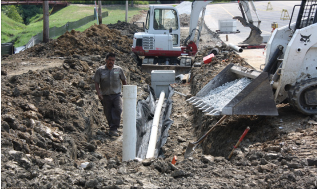
A system of underdrains and overflow outlets were installed along a 400 foot section of stream to promote infiltration and pollutant removal.
