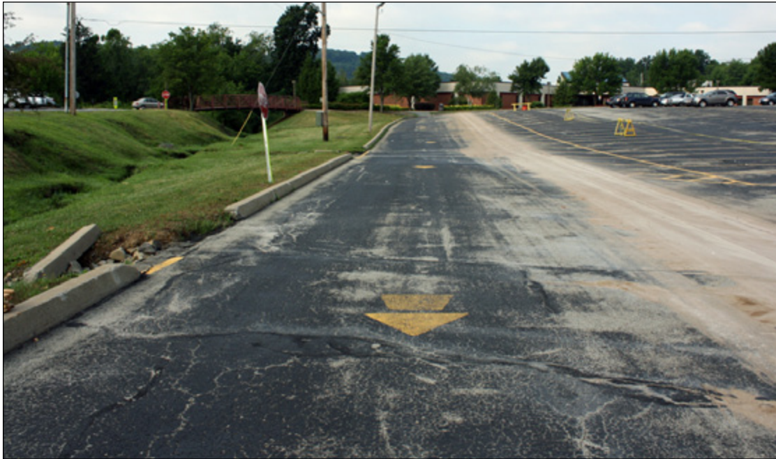
The Westmoreland County Community College had excess paving at the low end of a 4 acre parking lot that was within just 15 feet of the stream.
