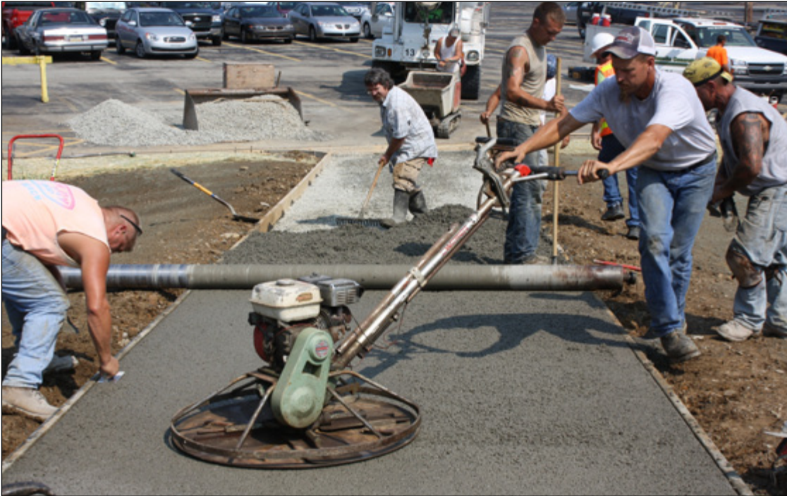
A new permeable concrete walkway, which will not produce stormwater runoff, connects the end of the pedestrian bridge to the parking lot across the widened riparian buffer.
