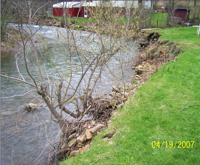
Streambank erosion on a bank section of Jacobs Creek next to a landowner's house and property
