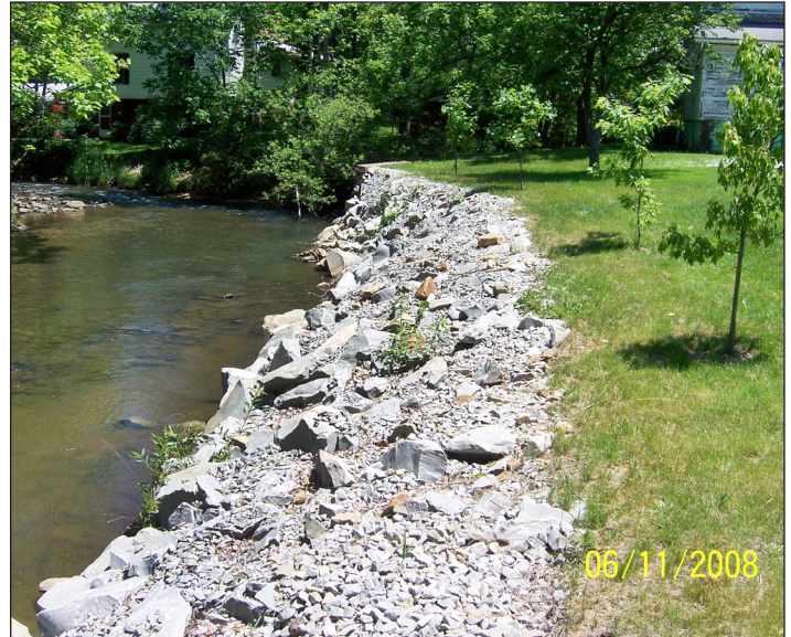
Installed rip-rap and riparian buffer on the same section a year after construction
