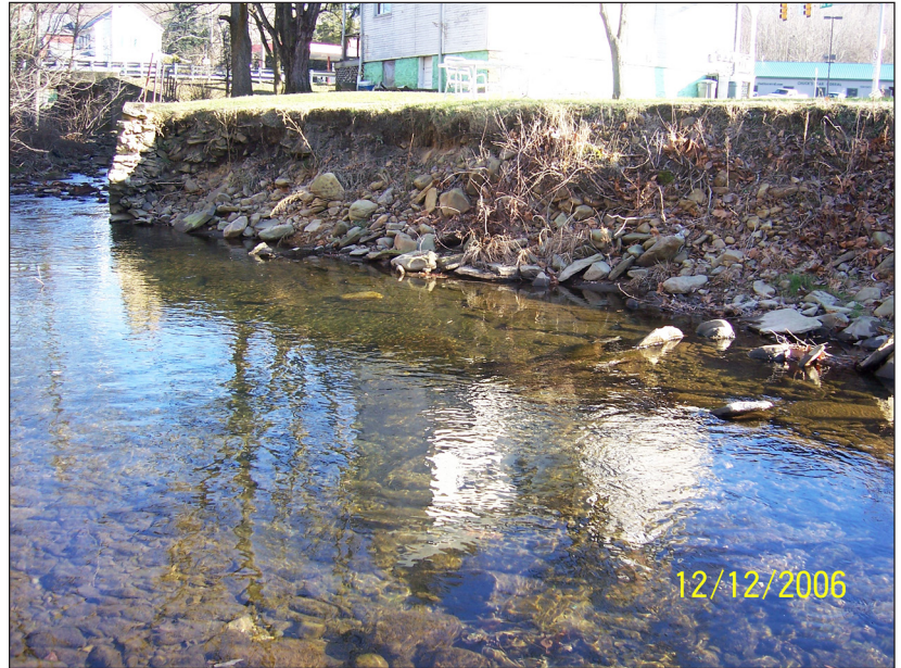
Severe streambank erosion on a section of Jacobs Creek
