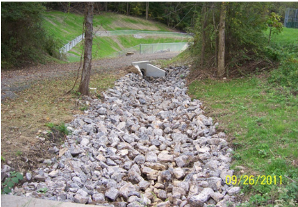
Site after construction with installed rock lined channel leading to the newly installed 400,000- gallon detention pond.
