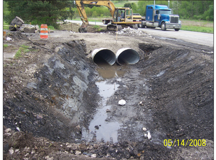
Installation of upgraded cross pipes at one of the four stream crossings
