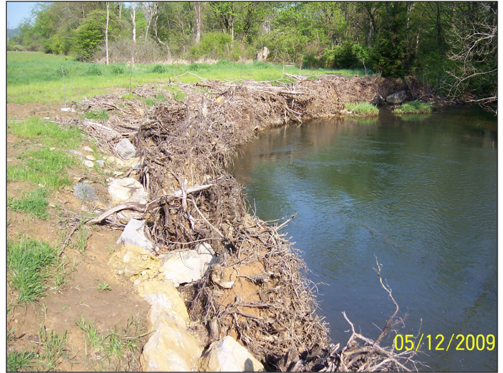
Rootwads and rip-rap installed along the same bank at the Denison property
