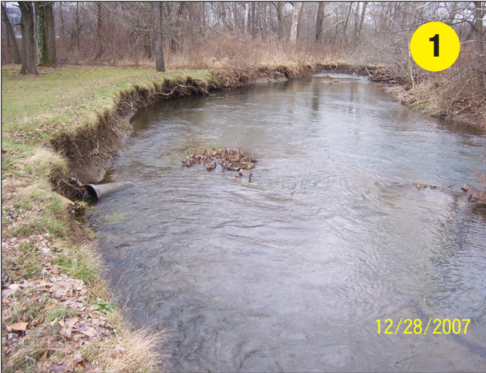
Another streambank along Mill Creek at the Denison property before any stabilization was done
