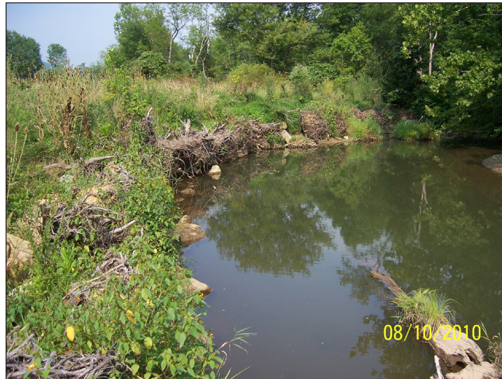
The bank section at Denison over a year later since the installation of the rootwads and rip-rap
