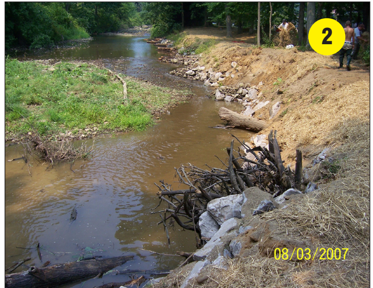
The streambank with rootwads, multi-log vane deflectors, and rip-rap installed. The bank is also being re-seeded.
