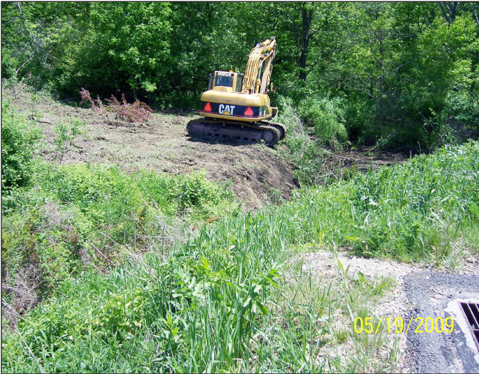
Area next to the Greenforge Office Building during construction of the stormwater retention basin
