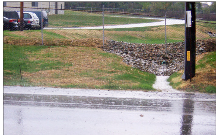
Bureau of Parks and Recreation site after construction with retention basin in place
