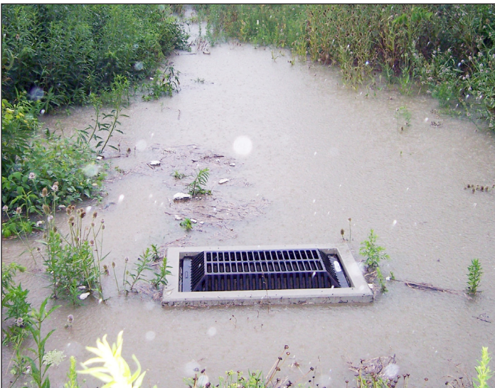
The retention basin managing stormwater during a rainfall two years after construction
