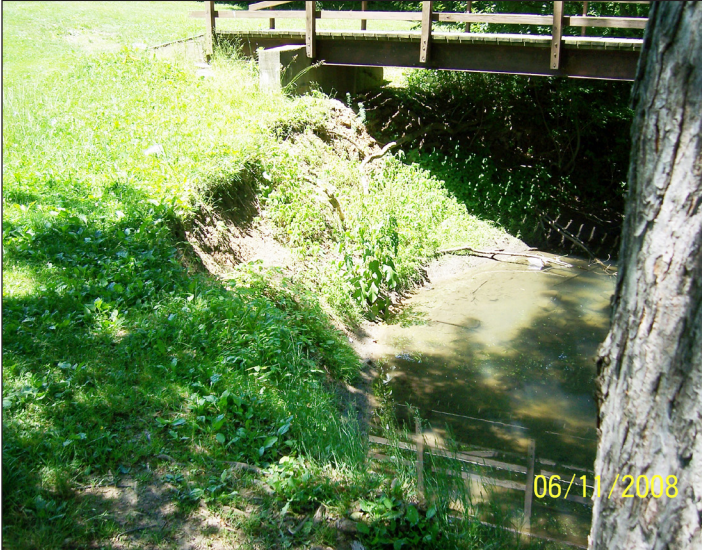
Eroding bank near pedestrian bridge
