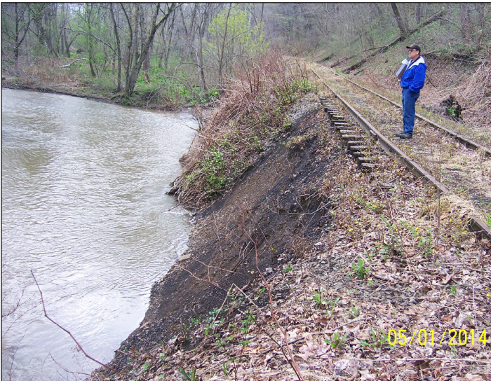
Stream bank before stabilization
