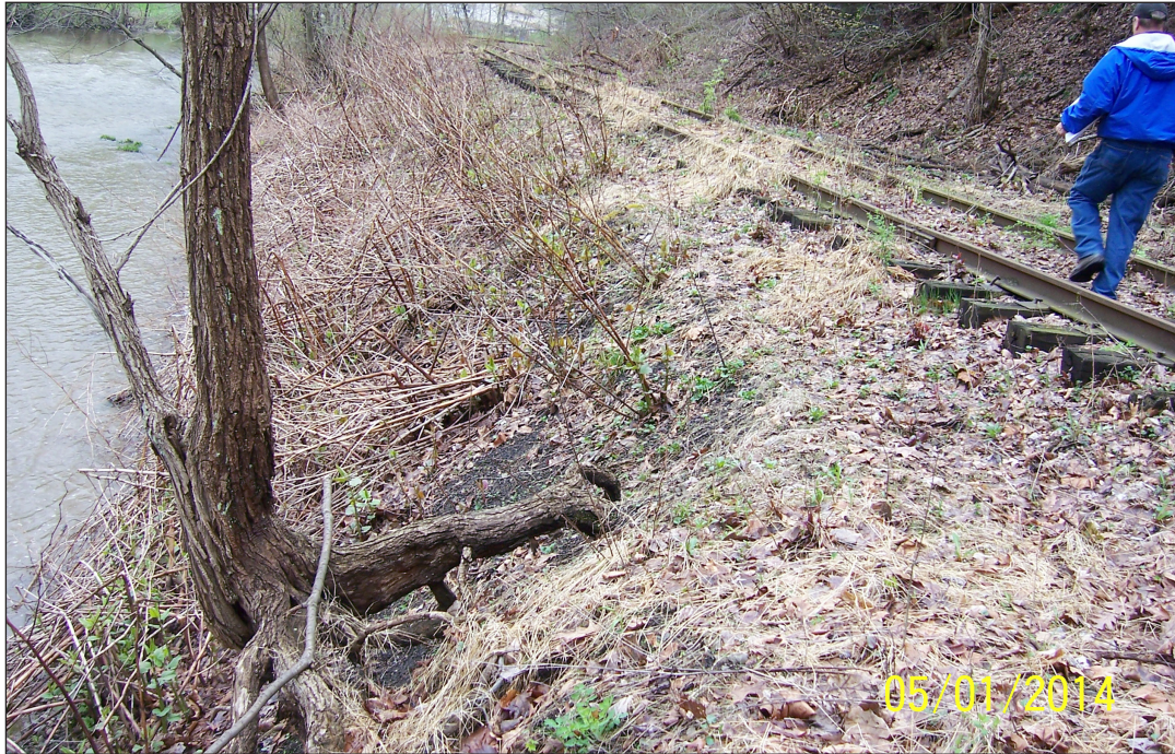
Note the exposed tree roots which are evidence of erosion
