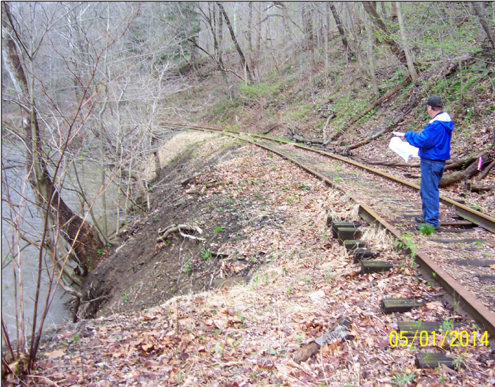
Eroding section of stream bank along what would become another section of the Westmoreland Heritage Trail
