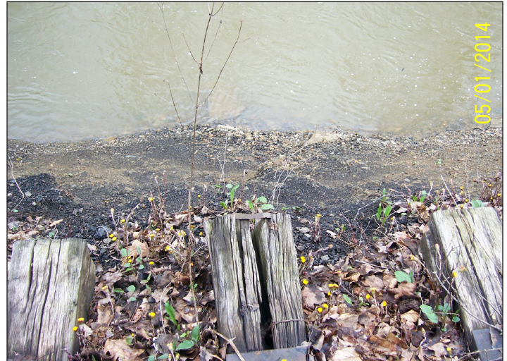
The erosion along Turtle Creek's banks was so severe on parts that it was beginning to undercut the railroad itself
