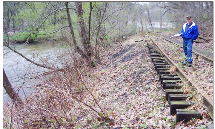
The exposed railroad ties are evidence of how much soil has eroded off of the banks
