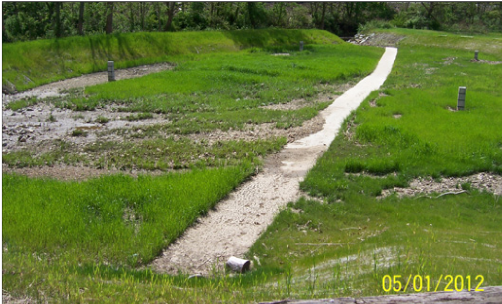
Constructed debris basin aids in the reduction of debris accumulating in the flood control channel in front of the school.
