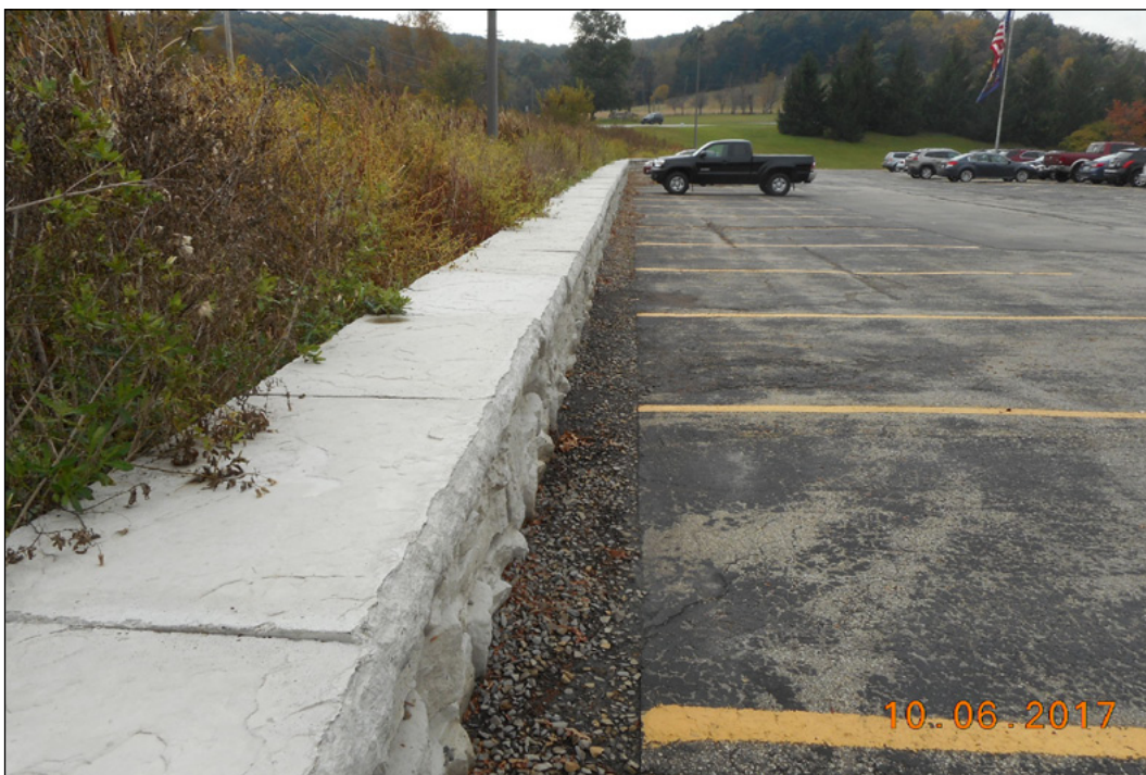
The same area after a Redi Rock wall was installed with underdrain, and the channel to the left was re-aligned
