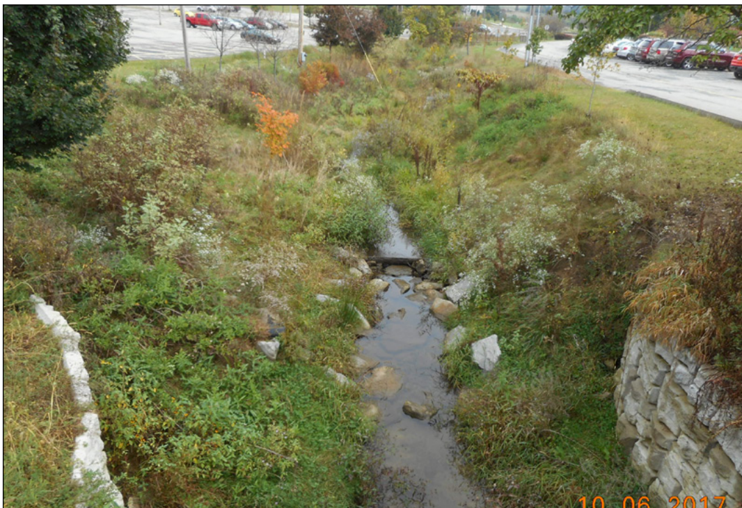
The same section a year after construction; Redi Rock was installed to stabilize the banks underneath the pedestrian bridge
