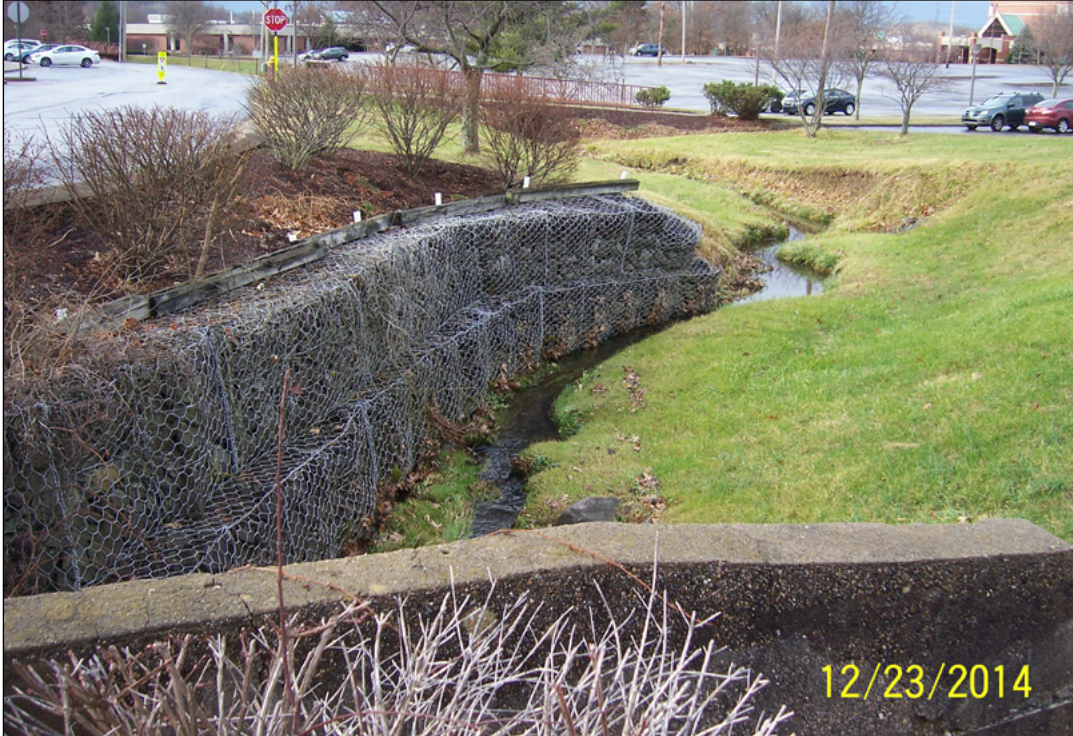
Moving downstream, the next section of Cherry Creek before construction; the gabion baskets were falling in on the end and again, the bank was being mowed to the edge
