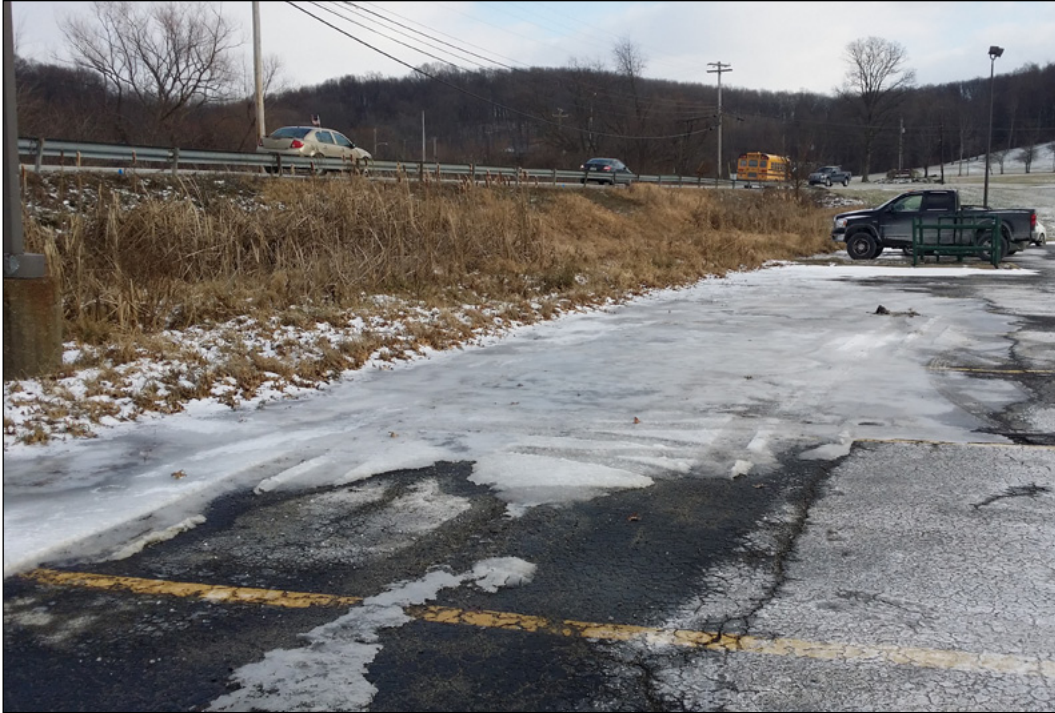
The parking lot area next to Armbrust road where the stream channel needed re-aligned; note the ice frozen over the parking spaces caused by the poor drainage
