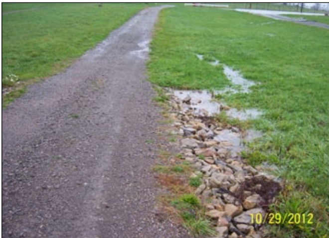
Picture taken during hurricane Sandy showing flowing water through road (French mattress) with no pipe!
