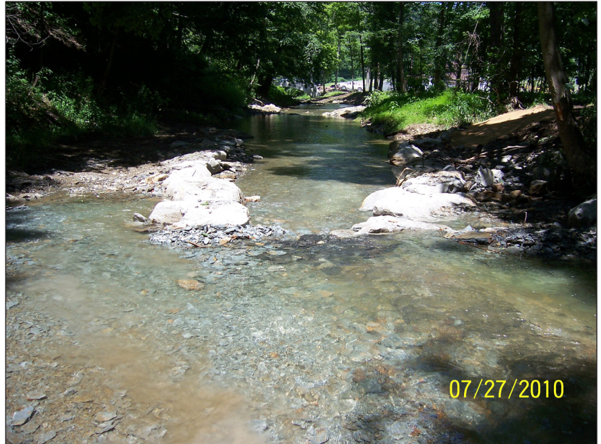
Rock cross-vane installed in the Chartiers Run to redirect the flow of water back to the center of the channel
