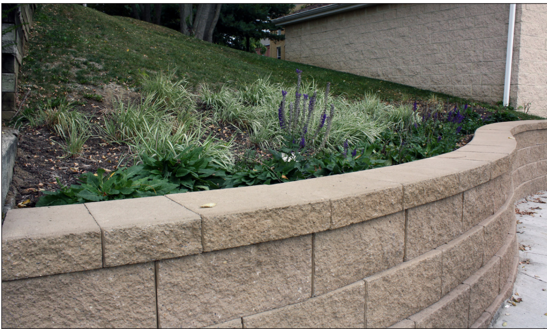
A rain garden behind a new retaining wall captures runoff before it gets to a heavily traveled pedestrian walkway and parking lot.
