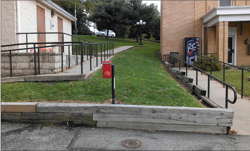
An existing timber wall holds back a slope where water pools and freezes in the winter, creating a hazardous condition in front of the Borough building.
