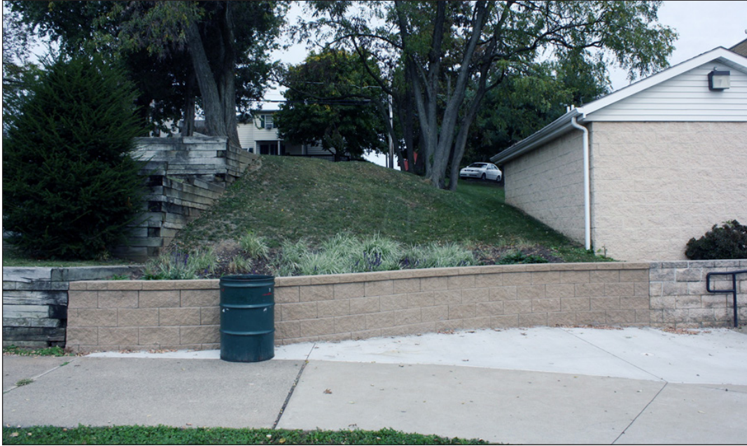
A concrete unit wall system holds back an existing hillside and the design layers of a rain garden.
