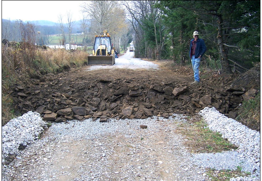
During construction: Raising the road profile and installation of underdrain on right and left side of road.
