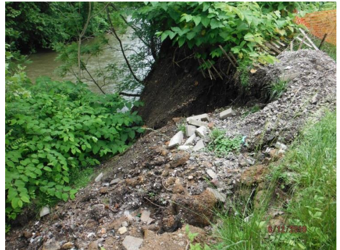
BEFORE CONSTRUCTION: Top of streambank. Note the loss of sediment and unconsolidated fill that has eroded into Loyalhanna Creek.
