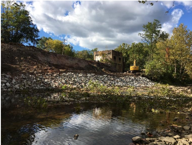
DURING CONSTRUCTION: Streambank terraced to allow for equipment to reach and place rip rap to armor toe of the slope.
