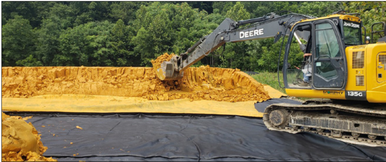
At the Lowber mine-discharge treatment site, an excavator is used to stir the iron sludge to speed its drying. Iron oxide is a pollutant that drops out of the mine water as it flows through the site's holding ponds. Periodically, it is removed from the ponds and stored on-site until it is dry enough to truck away.
