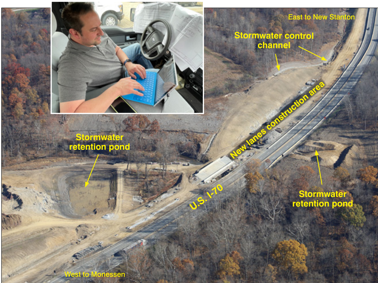
An aerial view of some of the most recent work on Interstate 70 that our senior erosion control specialist (pictured, inset) regularly inspected. This work disturbs massive amounts of earth, and our job is to help ensure that it does not get into local waterways.
