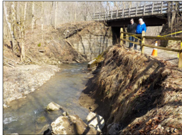
Severe erosion has worn some of Cedar Creek’s streambanks to within inches of the blazed trail in the county park of the same name. In 2020, we received funding to stabilize and rebuild about 900 feet of those banks. That work is planned for 2021.
