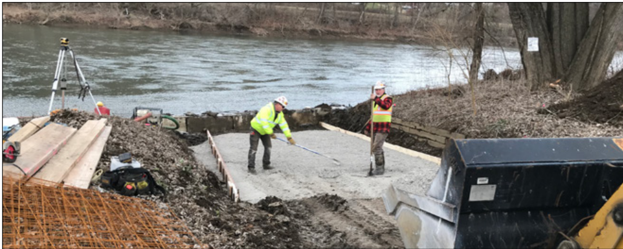
With several partners, we were able to create a new concrete access to the Youghiogheny River in West Newton, which will significantly reduce erosion from this very popular boat launch area.
