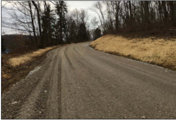
Brown Road in Allegheny Township is no longer essentially a one-lane road with dangerously steep berms. Trees were removed, and the bank on one side of the road cut back (right side in photo) to make the road wider. The road surface also was raised and a number of measures were installed to manage stormwater.
