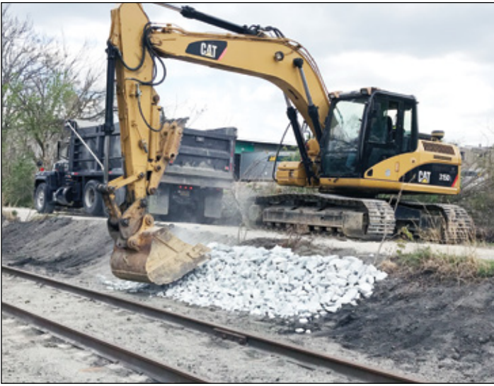
Stabilizing part of a slope with stone rip rap along the trail between Huff Avenue and Fairview Street in South Greensburg.
