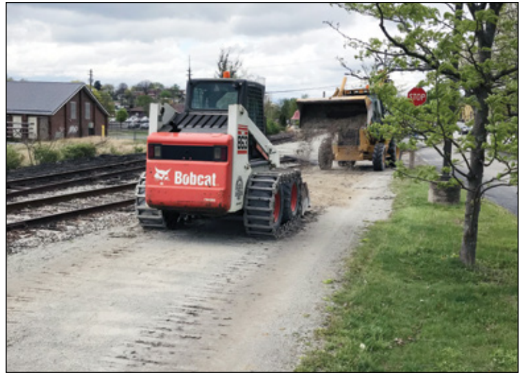
Resurfacing a section of the trail between Huff Avenue and Fairview Street in South Greensburg.
