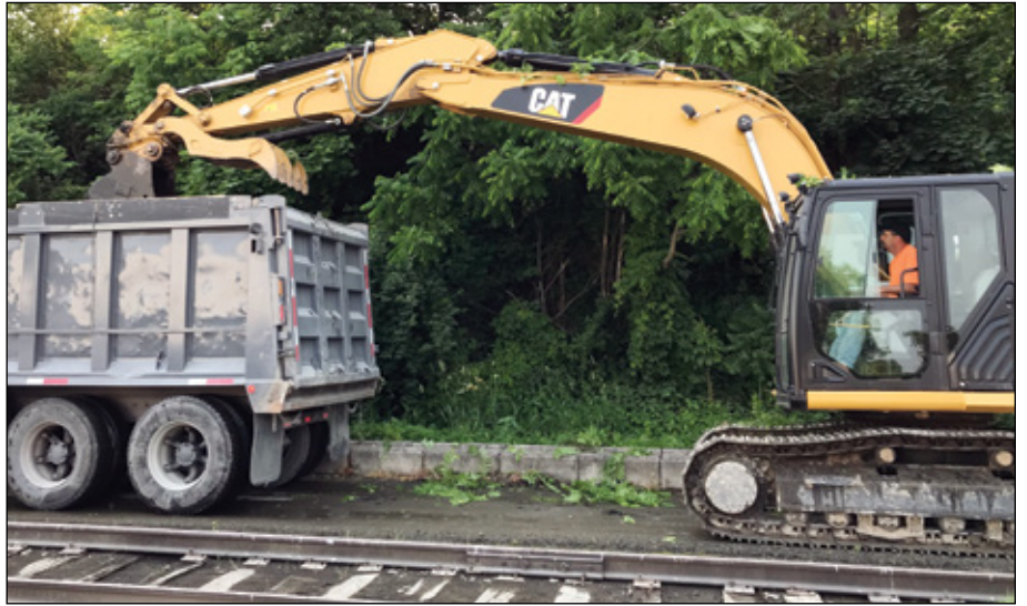
Loading the drainage channel sludge which will be hauled away and disposed of.
