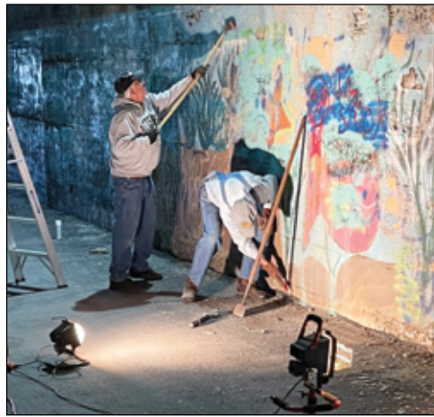
Bright shop lights strung through the tunnel helped everyone see what they were doing.
