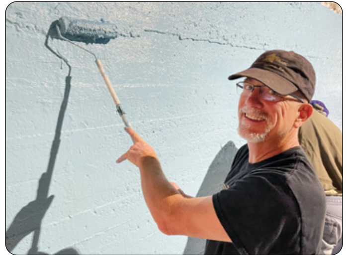
Five Star Trail President Vaughn Neill works as part of the great volunteer team who applied the blue undercoat paint over the primer in preparation for the new mural artwork to be painted in the tunnel near Lynch Field in The City of Greensburg.
