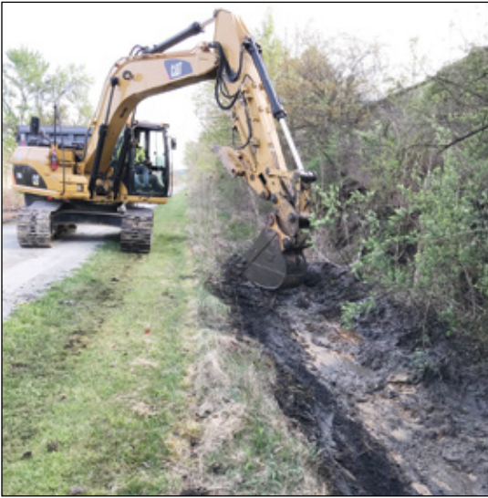
Opening a clogged drainage channel on the northern trail section near Lynch Field.
