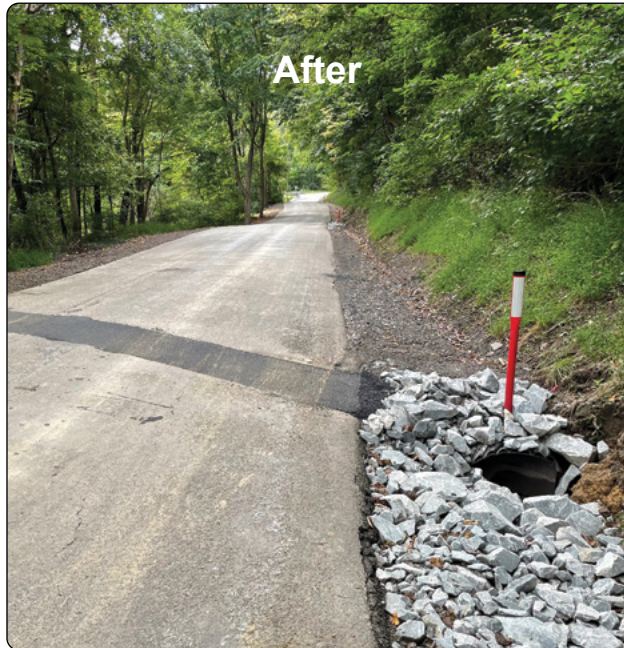
Multiple cross pipes were installed diverting the springs and road runoff under the road to a stable outlet.
