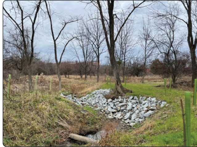
The stabilized unnamed tributary to Monastery Run.
