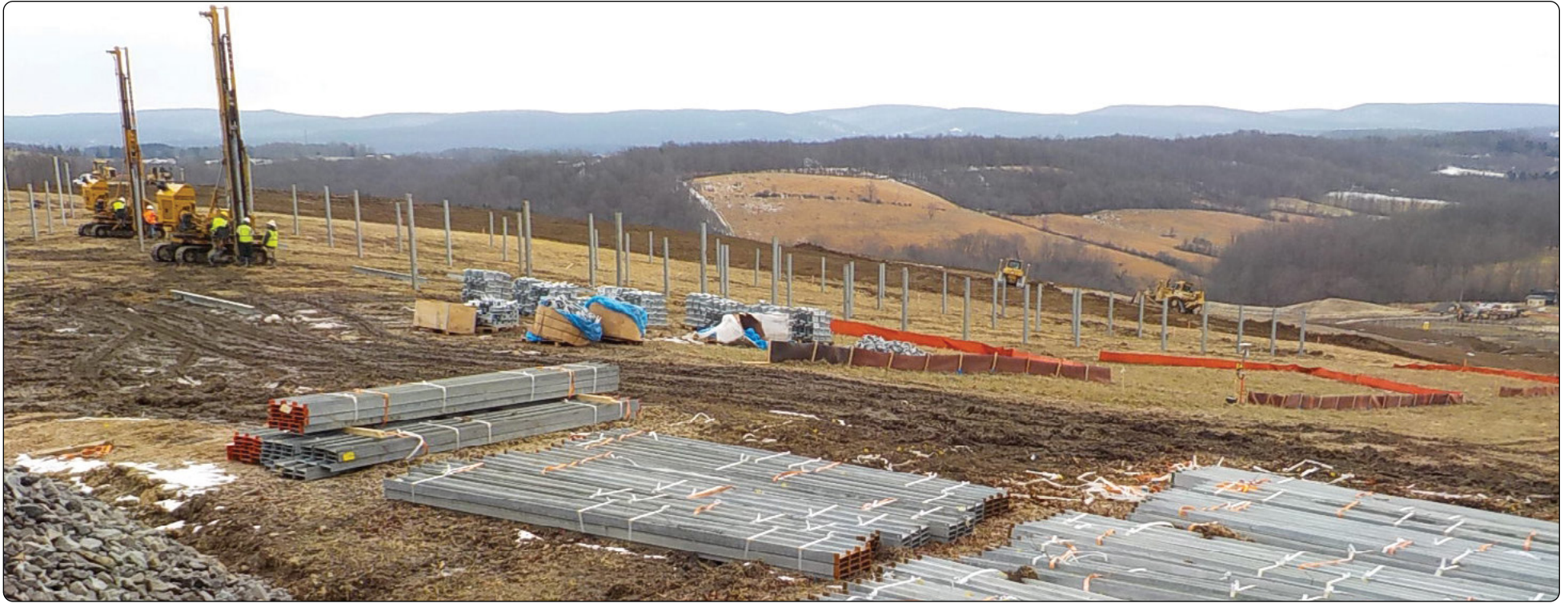
The steel post installation equipment drives posts into the ground at the new solar farm site. The view of the ridge and countryside from here is remarkable. Due to the slope of the hillside, extra caution is needed to help control soil erosion caused by earthmoving during construction.
