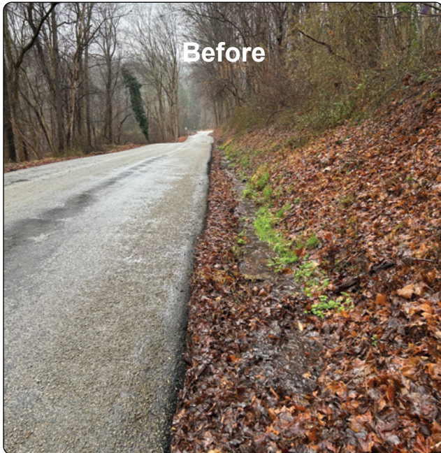
Multiple springs and road runoff causing water to flow down the road edge creating unstable and eroding ditches.
