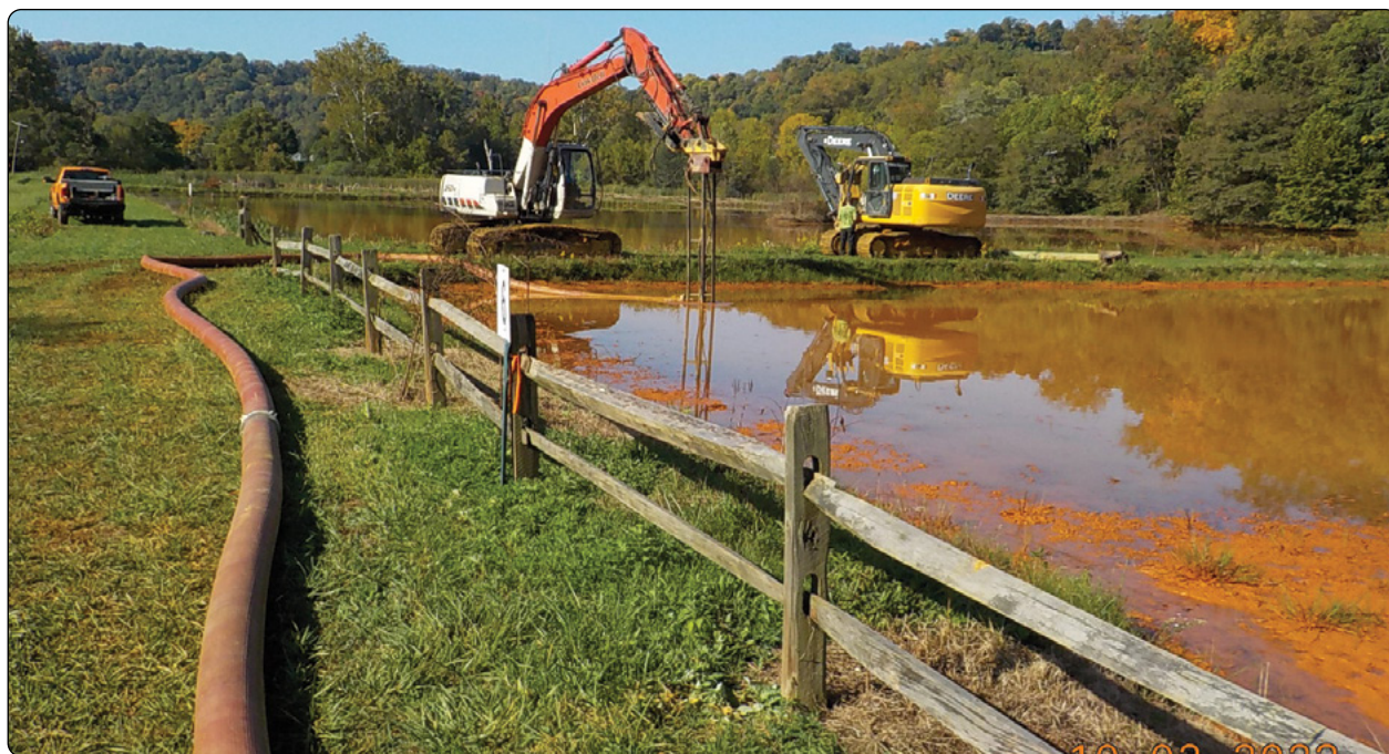
Pumping iron oxide sludge from the Lowber settling ponds to the giant containment bags.
