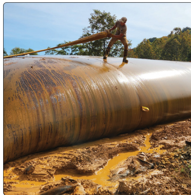
Recovered/removed iron oxide sludge pumped into these giant bags will be dried and prepared for sale to industries.
