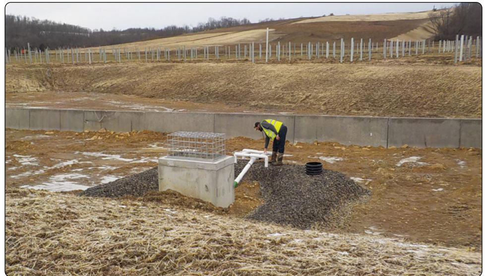
Inspecting a skimmer installed in a sediment basin at the bottom of the solar farm hill.
