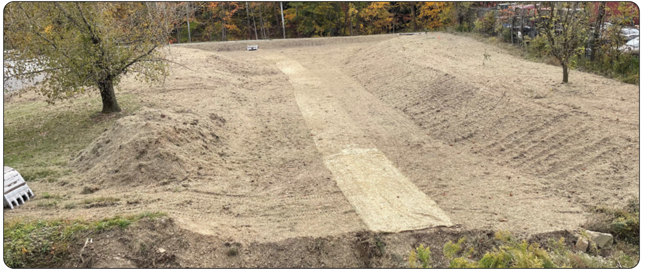
Newly constructed detention pond where large rain events will enter the pond and filter out pollutants before entering Turtle Creek.
