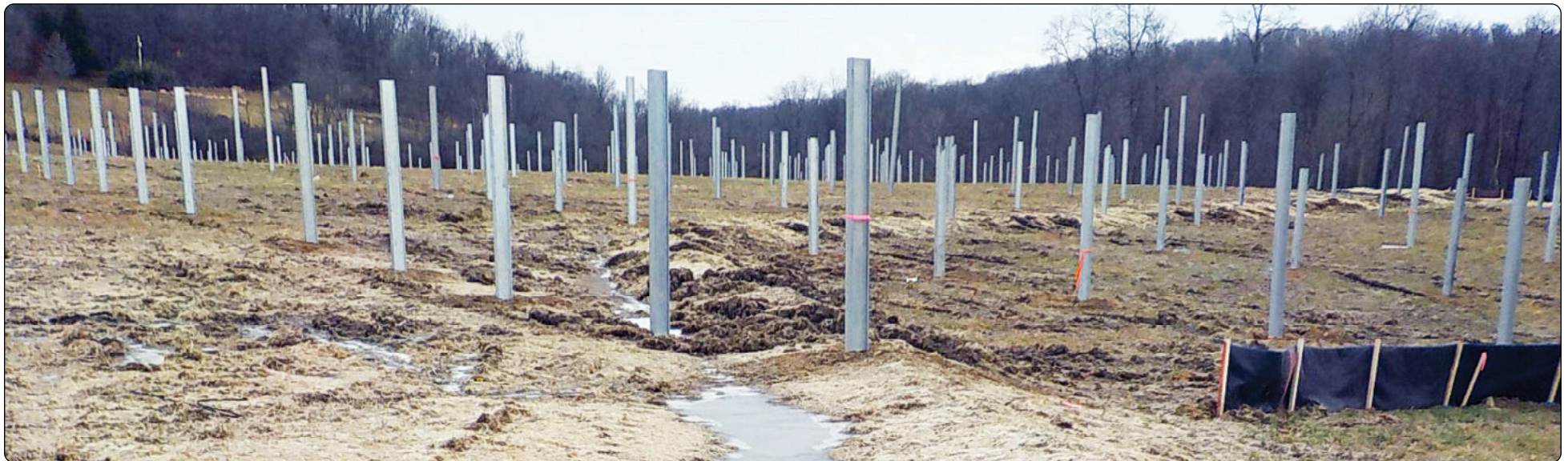
This forest of steel posts will soon be supporting the panels for the largest solar panel farm to date in Westmoreland County.
