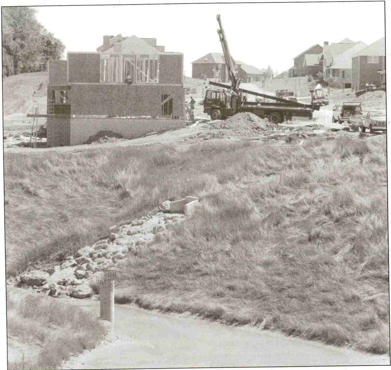
Conservation measures like this rock channel and basin help control the loss of soil on construction sites such as this one in North Huntingdon Township.
