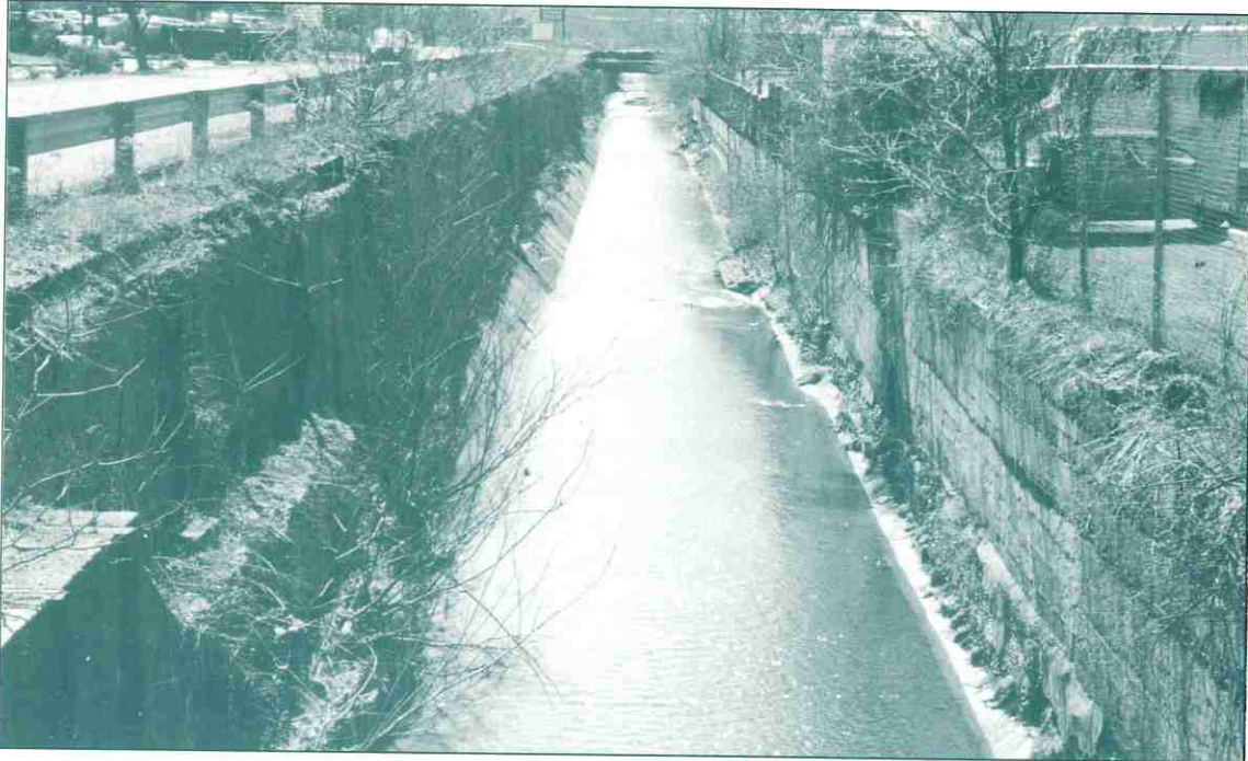
The old-fashioned way to control stormwater — Walworth Valve Company's flood control channel in South Greensburg, on Jack's Run.
