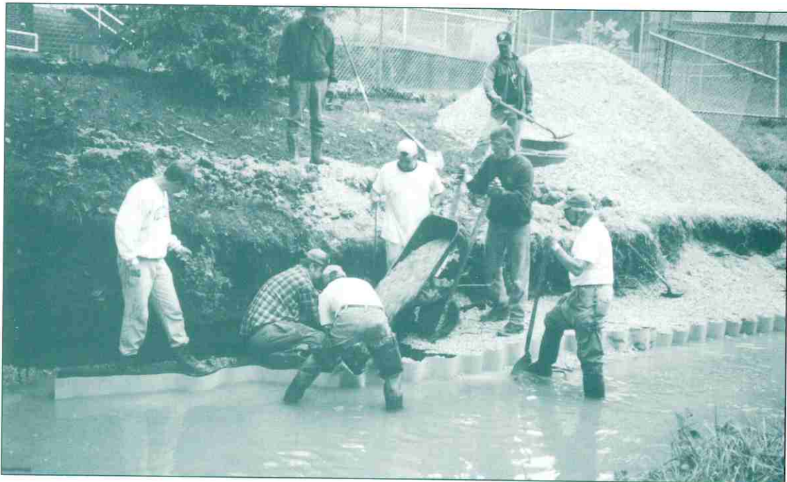
Volunteers work to install low-cost, environmentally friendly streambank stabilization on Jack's Run at Lynch Field, City of Greensburg.
