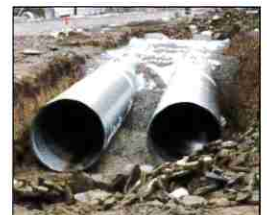
Underground retention tanks are one way of reducing the volume of runoff, but they do not improve the water's quality.
