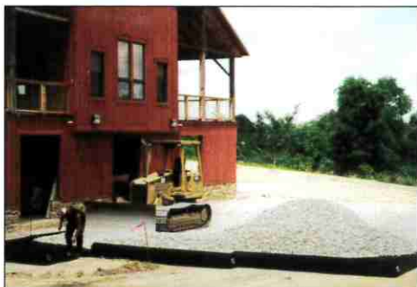
The crushed stone parking lot behind our Barn uses a geotextile layer to keep the stone clean and optimize infiltration of rainfall.
