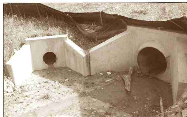
Discharge of sediment from a malfunctioning sediment basin. Sediment pollution has occurred at this earthmoving site which will impact the waters of the Commonwealth.
