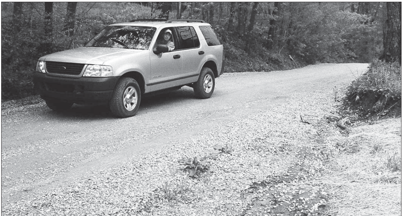
Mike Barrick, watershed specialist for the Westmoreland Conservation District, inspects work done on Firetower Road. The straw in the right foreground helps to prevent erosion from water runoff.
