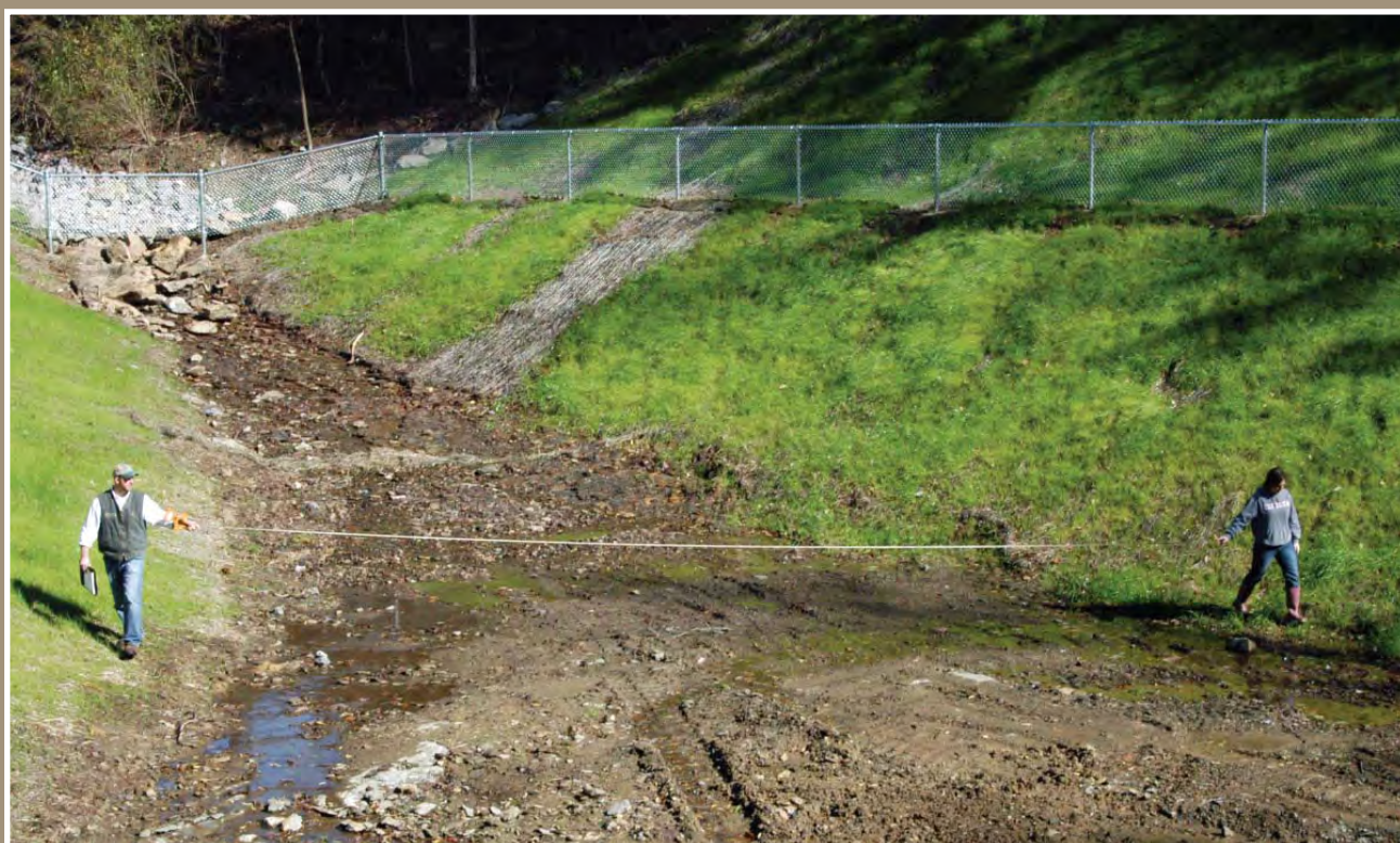
District Watershed Specialist Rob Cronauer (l) and Intern Samantha Pedder (r) measure the nearly completed Kinloch Basin. It has a 400,000 gallon capacity and is one of the largest stormwater basins the District has ever built. See page 17 for more information.
