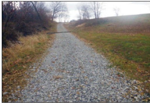
A long, steep access road on private property in New Alexandria shows the damaging effects of unmanaged water runoff (top) and (bottom) conservation improvements implemented by the owner after attending the District's driveway workshop.
