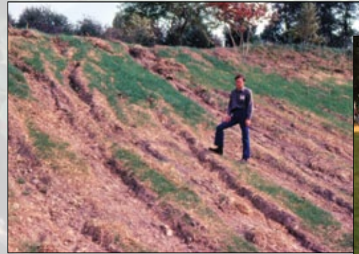
1980 – All it took was one bad thunderstorm to carve gullies and create severe erosion in steep slopes like this one at Newhouse Park in Delmont.
