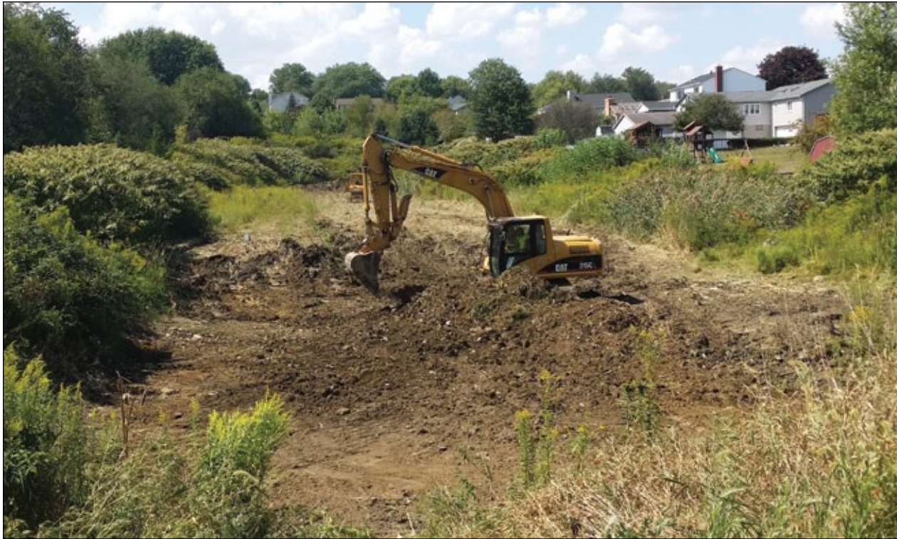
Work continued on a multi-year effort to help municipalities improve the functioning of older stormwater ponds, including this one in Penn Township. Well-functioning stormwater ponds help reduce the risk of flooding and benefit water quality.
