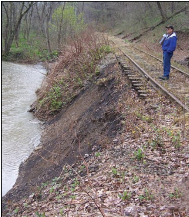
One of the severely eroded streambanks along Turtle Creek that will be stabilized with rip rap and trees, thanks to a grant received in 2015. This area will become the base for the Turtle Creek Trail extension of the Westmoreland Heritage hiking/biking Trail.
