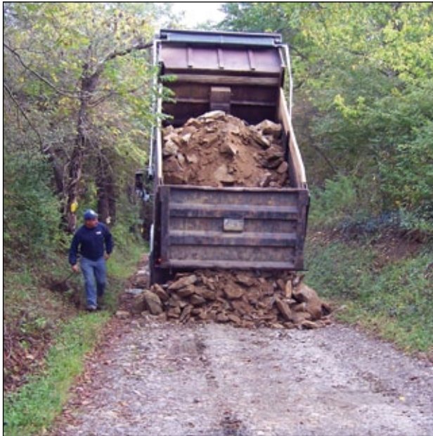
Portions of Misty Meadow Road in Mount Pleasant Township were so severely eroded that they were as much as three feet below the level of the surrounding ground. More than 100 tri-axle truckloads of shale rock were needed to build the road surface back up.
