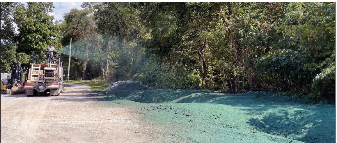
Hydroseed is sprayed on infiltration swales for final stabilization at Irwin Park.
