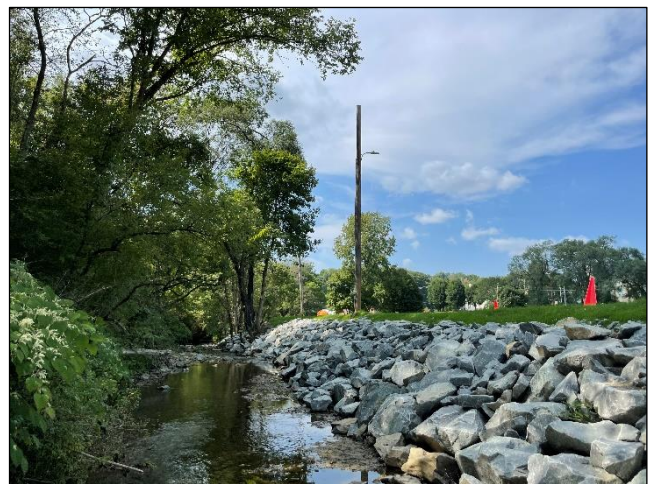
(After) Banks graded back to a stable slope and rock added to the toe of the slope.
