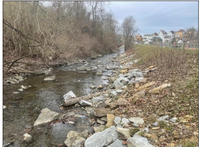
(After) Banks graded back to a stable slope and single log vane deflectors (10) installed to stabilize eroding streambank.
