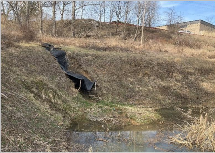
(Before) Existing plastic channel as outlet to basin with accumulated sediment.
