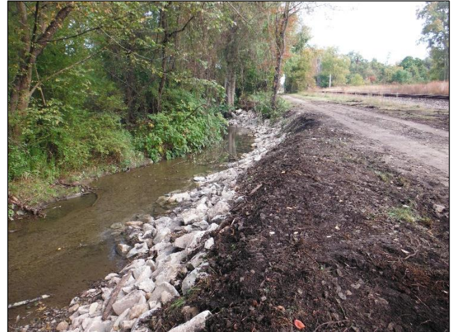
After: Banks graded back to a stable slope and rock saw-tooth deflectors installed along the toe of the slope
