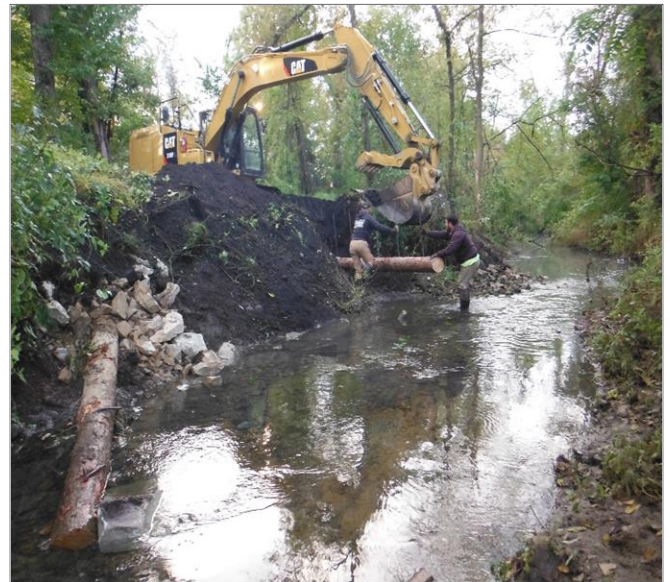
Single log vane deflectors being installed to help direct stream current away from stream banks
