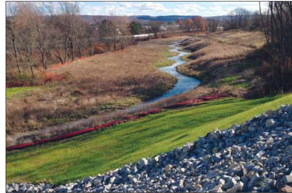
The newly relocated section of Sherrick Run in Mount Pleasant Township, Jacobs Creek Watershed, is shown here just a few months after construction of a 100-plus-foot riparian buffer with micropools and plantings for habitat and wildlife, both of which also will help to protect water quality.
