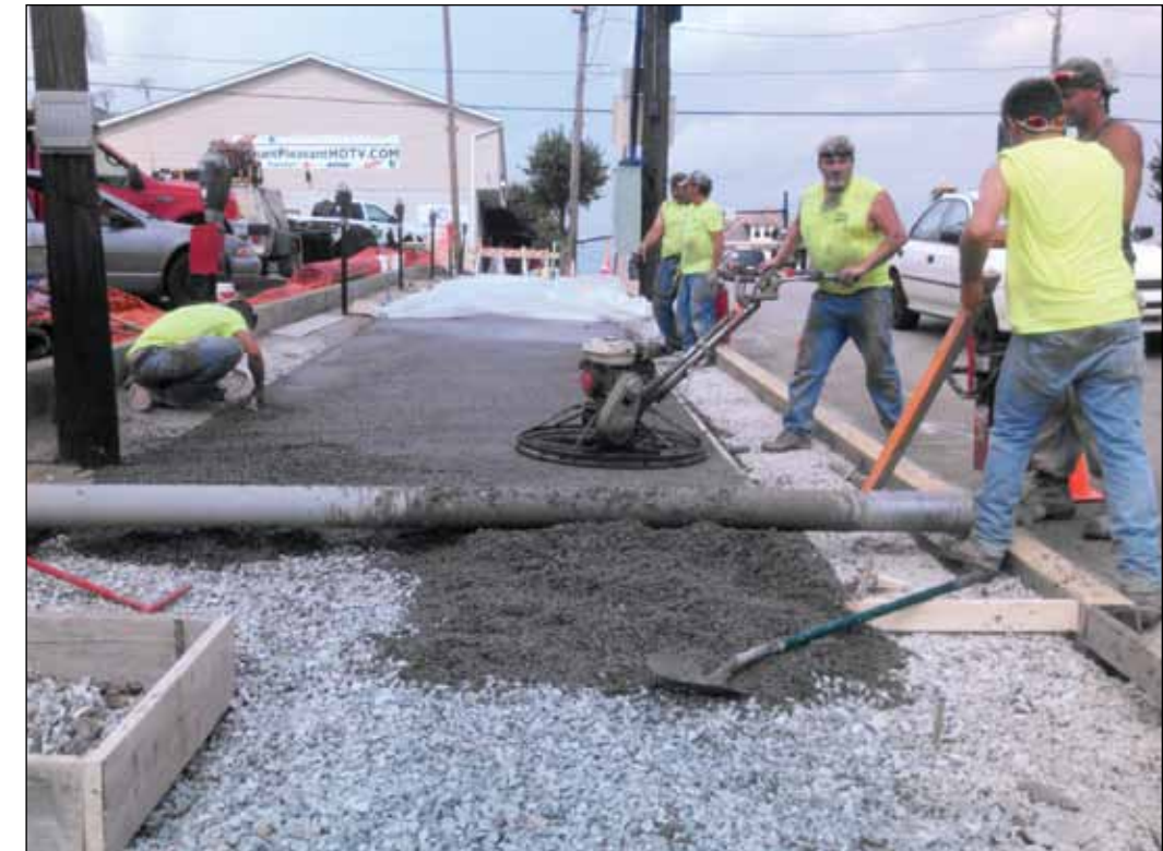
Contract workers install a porous concrete sidewalk over a stone and perforated pipe infiltration bed along Diamond Street in Mount Pleasant Borough, Jacobs Creek Watershed. Trees also were planted here and will be watered as rain and melting snow and ice infiltrate through the sidewalk.
