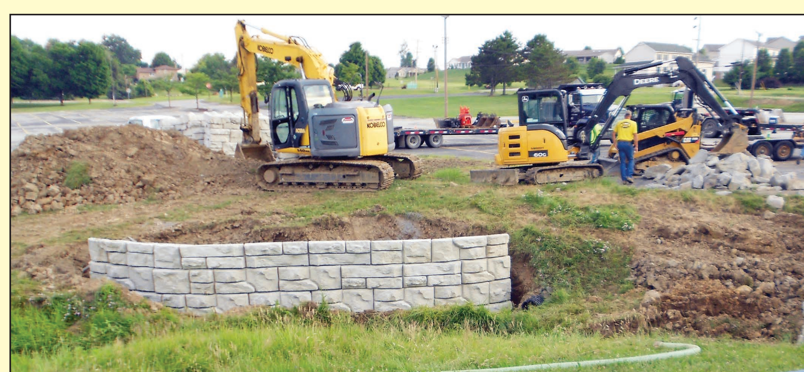
Ramsey Excavating placed a retaining wall along Cherry Creek, part of a larger riparian buffer project at Westmoreland County Community College in Youngwood.
