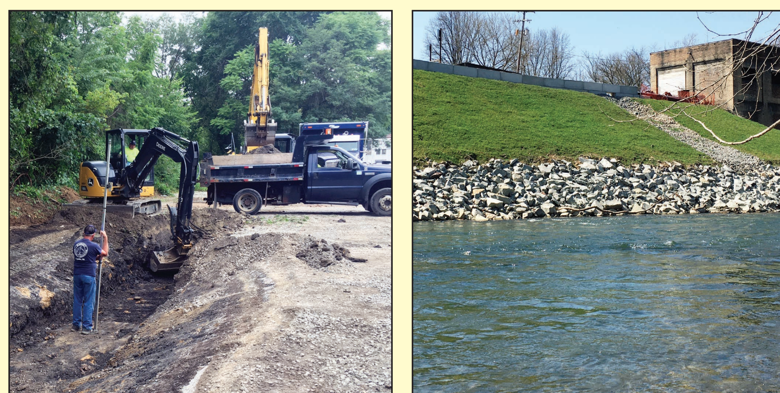
(l) In Irwin, the company excavated for a rain garden to capture runoff from a parking lot. (r) Ramsey's stabilization work along the banks of the Loyalhanna Creek in Latrobe.
