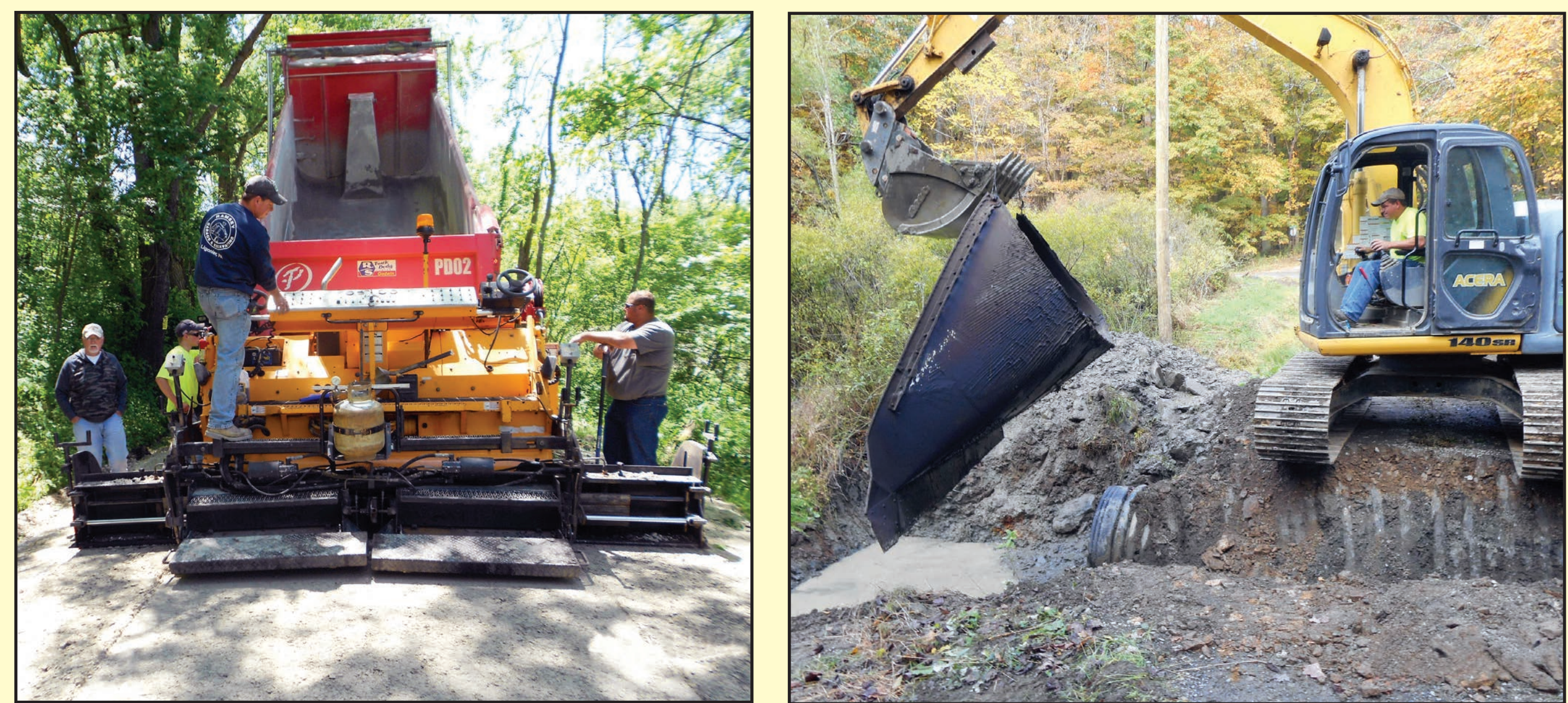
(l) Ramsey Excavating paved Misty Meadow Road in Mount Pleasant Township with diving surface aggregate. (r) In a project in the eastern part of the county, Bobby placed a flared-end section of squash pipe to carry the full width of a stream.
