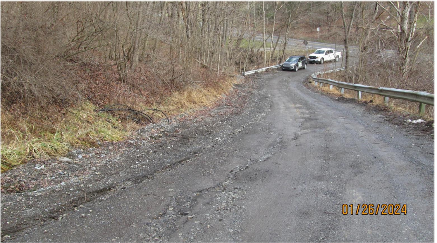
(Before): Unstable gravel surface and eroding ditches
