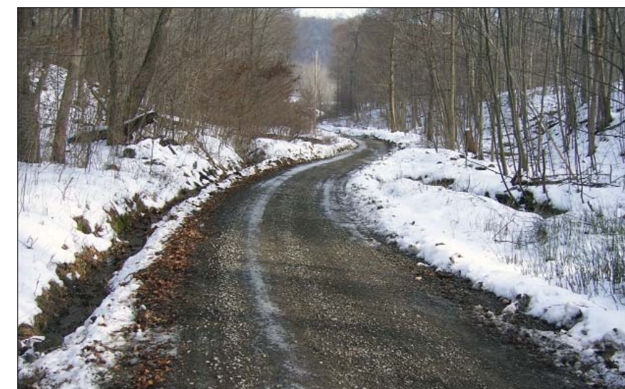
Because it was so badly eroded, Keiper Road was almost like a streambed – the low point where water would collect.
