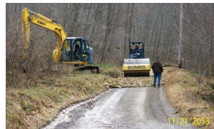
Improvements included raising the road surface as much as three feet. Pipes and underdrains will also be added and the combined effect will be to keep as much water as possible off the road surface.
