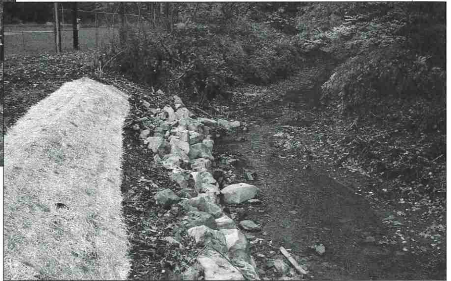
Right: Phase One improvements, completed this fall, slowed erosion by stabilizing the streambank near Valley High School's athletic fields.
