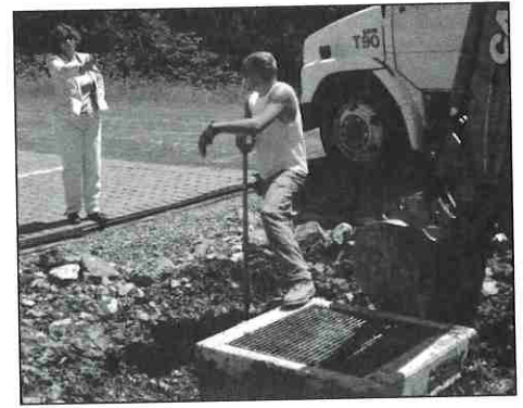
District Landscape Architect/Stormwater Technician Kathy Hamilton supervises the installation of a stormwater demonstration best management practice at GreenForge.
