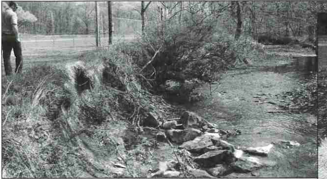
Above: Little Pucketa Creek's channel has lost capacity over the years due to soil eroding from the streambanks.
