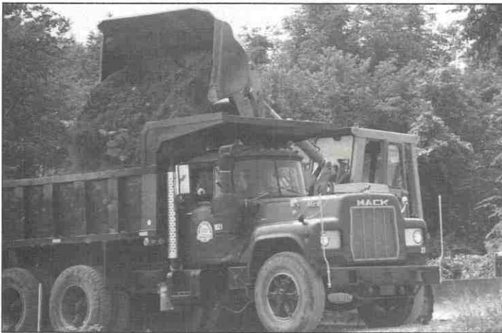
Adam Eidemiller, Inc., donated men and equipment to excavate over 1,000 tons of earth for the barn.
