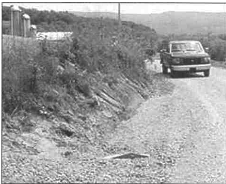
New catch basin on Frye Road, Derry Township, controls runoff.
